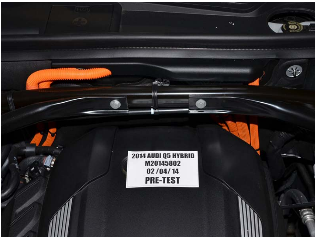
FIGURE 18d. Pre-Impact View of High Voltage Interconnect(s)
