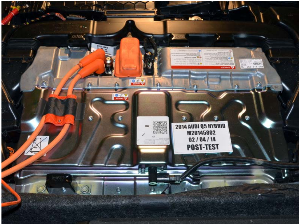
FIGURE 10. Post-Impact Front View of Propulsion Battery
