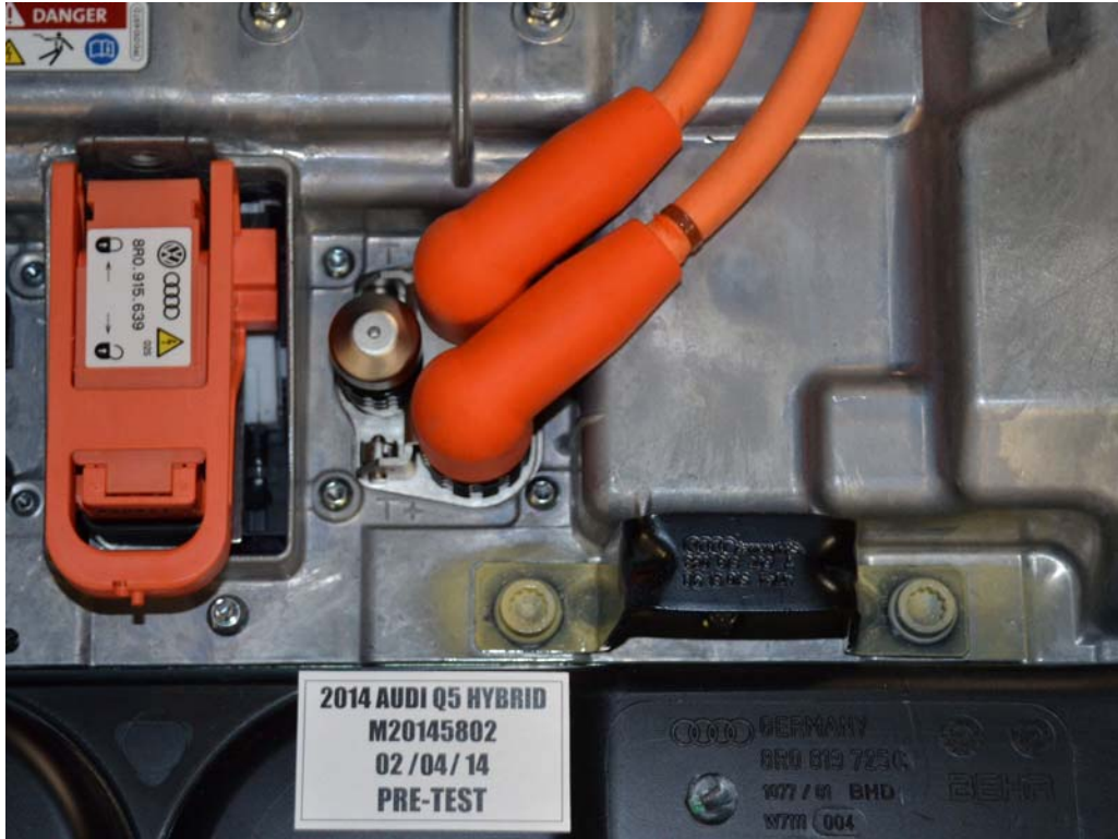
FIGURE 23. Pre-Impact Close-Up View of High Voltage Leads Attached
