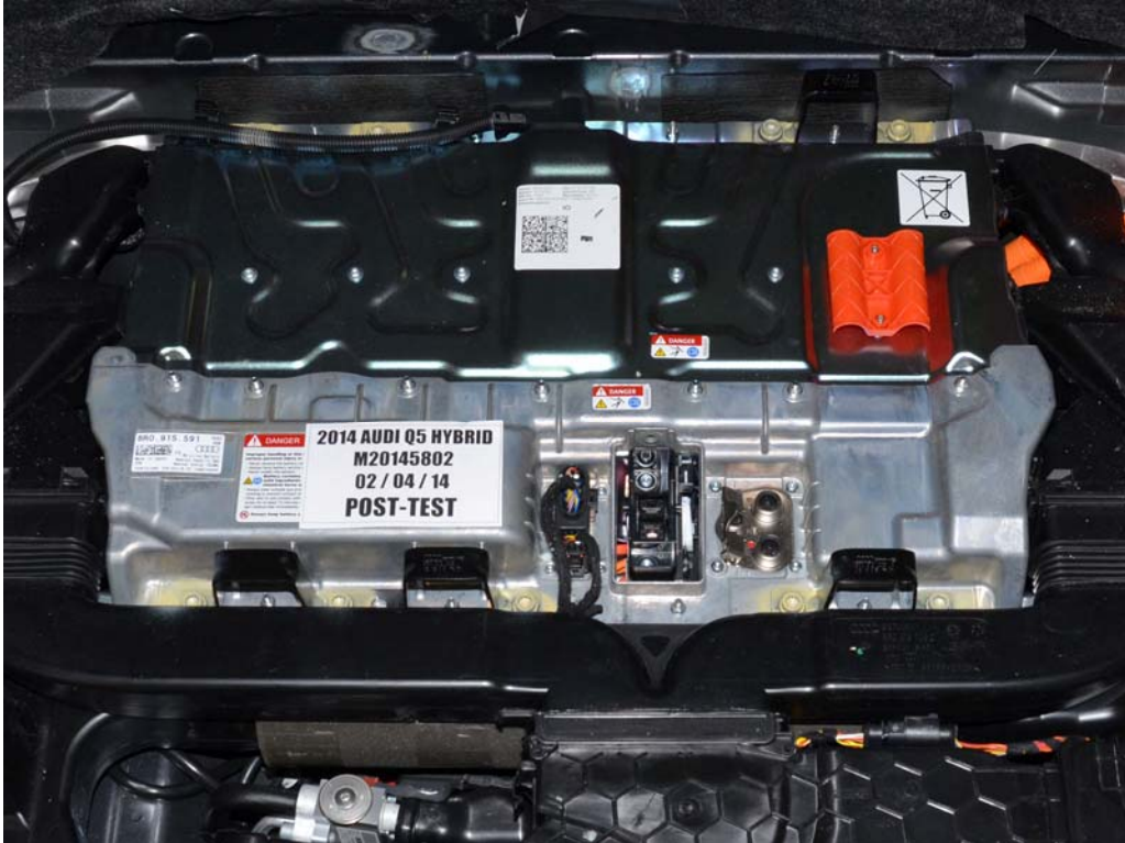
FIGURE 11. Post-Impact Rear View of Propulsion Battery
