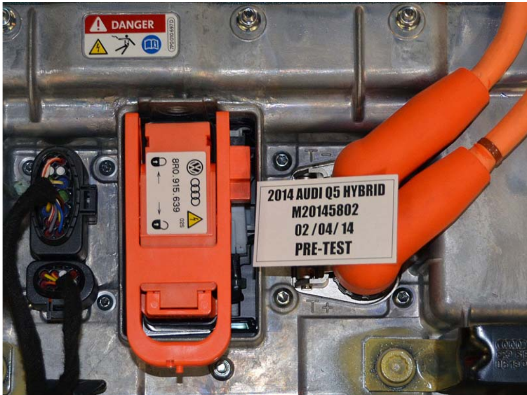
FIGURE 6. Manual High Voltage Service Disconnect in Place
