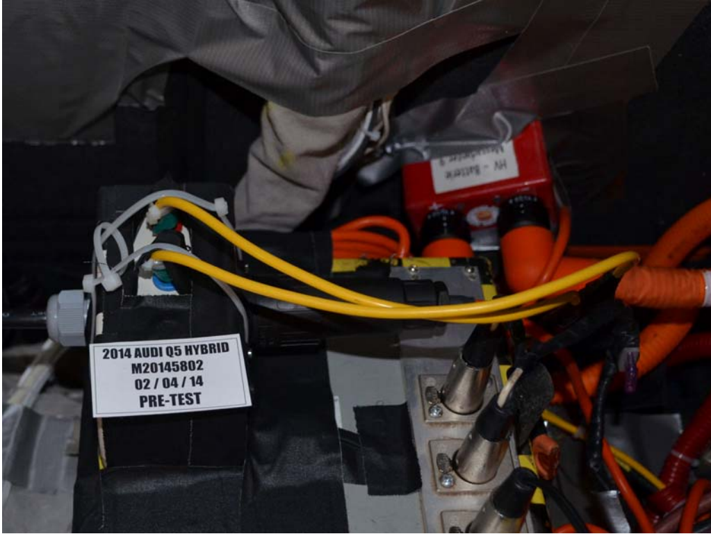
FIGURE 23b. Pre-Impact Close-Up View of High Voltage Leads Attached
