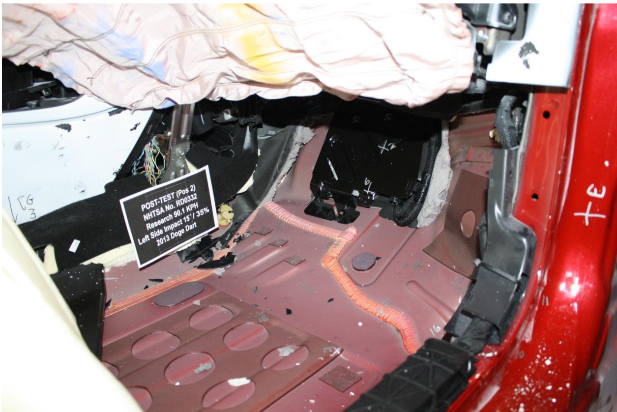
No. 093 Post-Test View of Passenger Floor pan at Left sill level, w/o carpet
