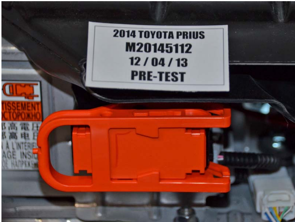
FIGURE 6. Manual High Voltage Service Disconnect in Place
