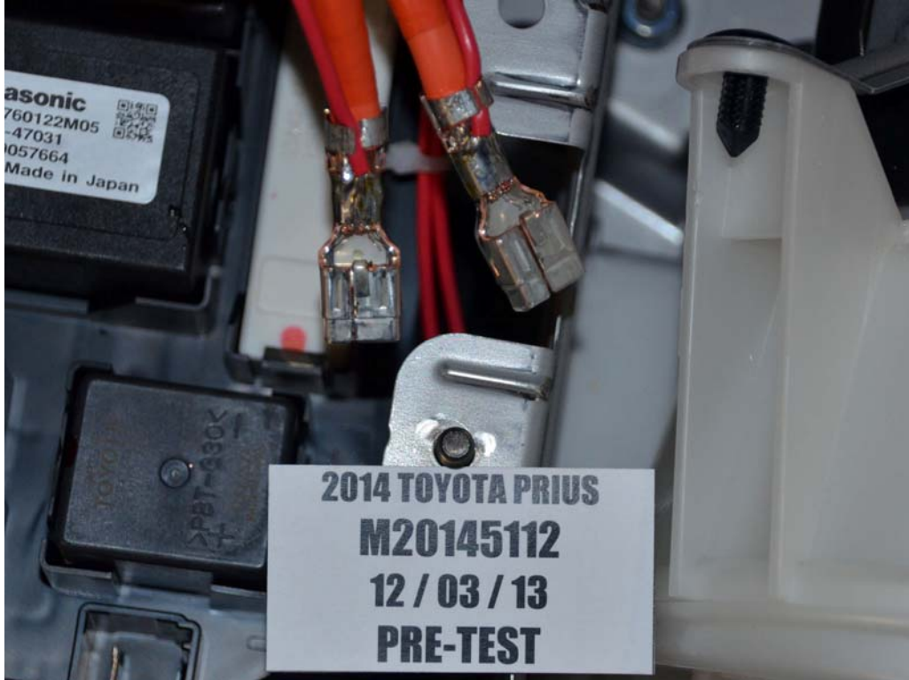
FIGURE 23a. Pre-Impact Close-Up View of High Voltage Leads Attached
