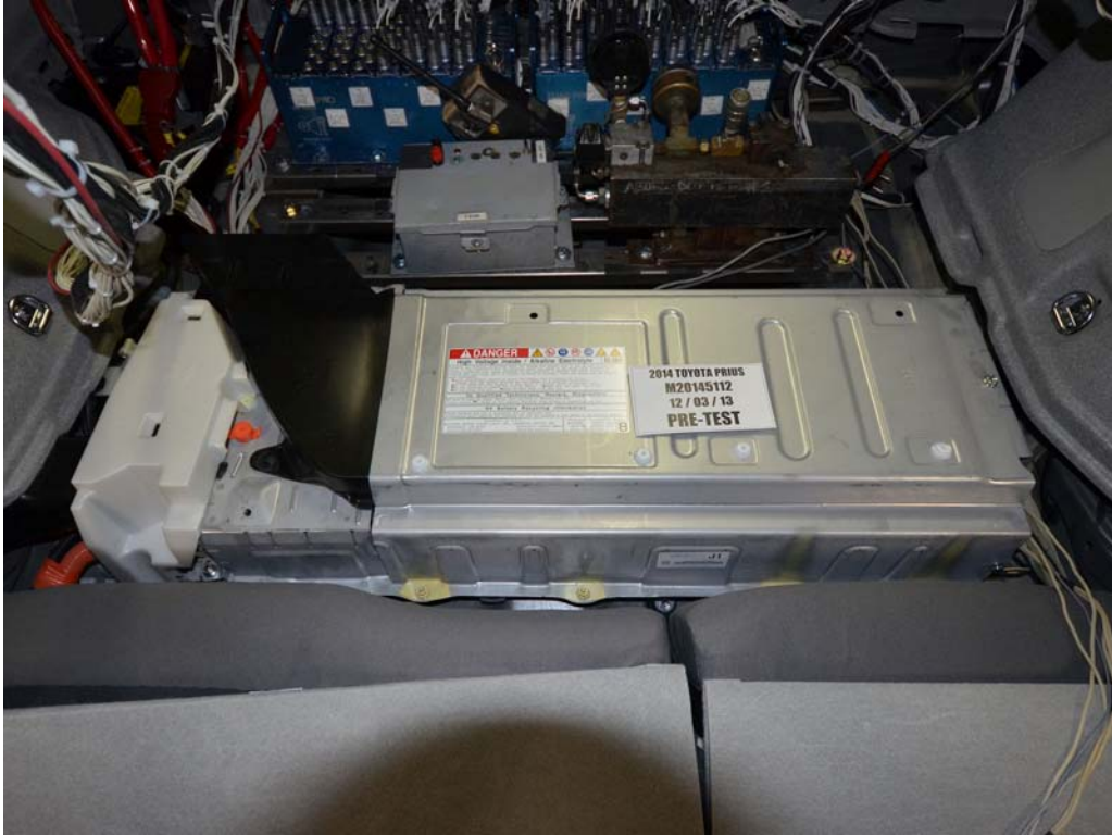
FIGURE 9. Pre-Impact View of Propulsion Battery
