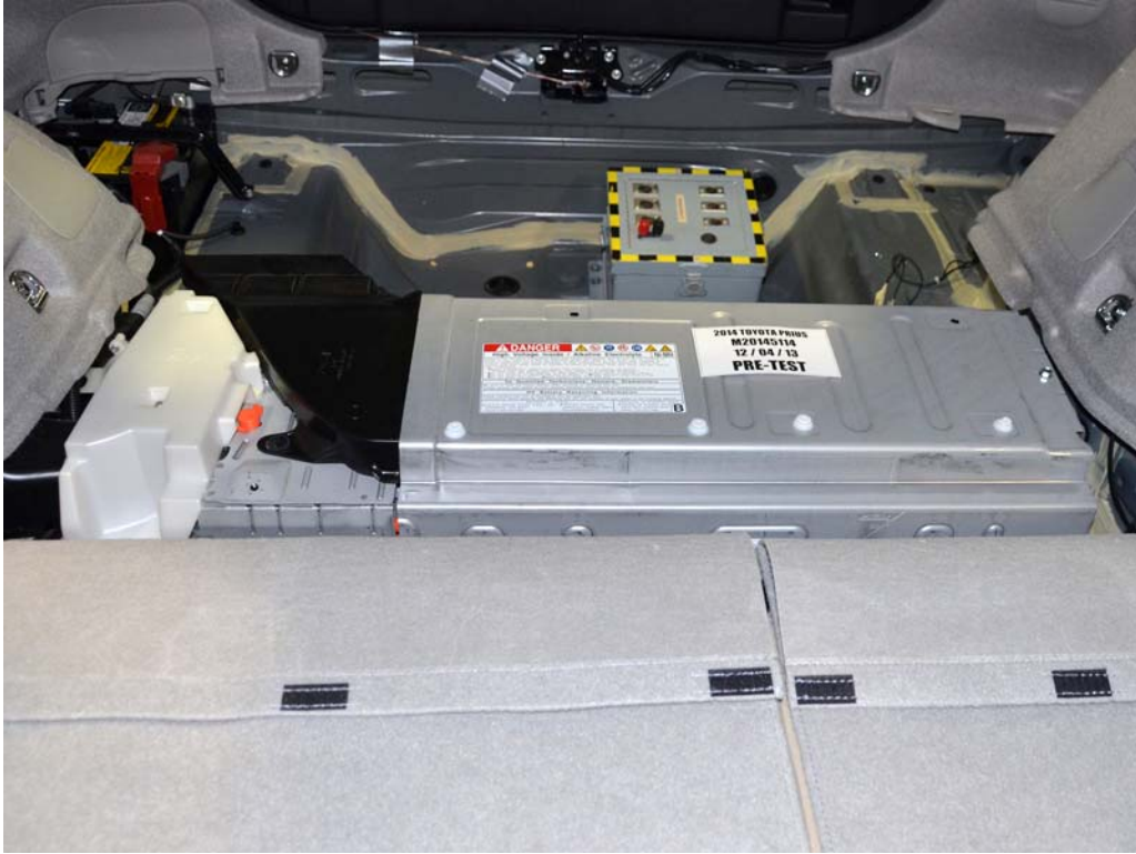
FIGURE 9. Pre-Impact View of Propulsion Battery
