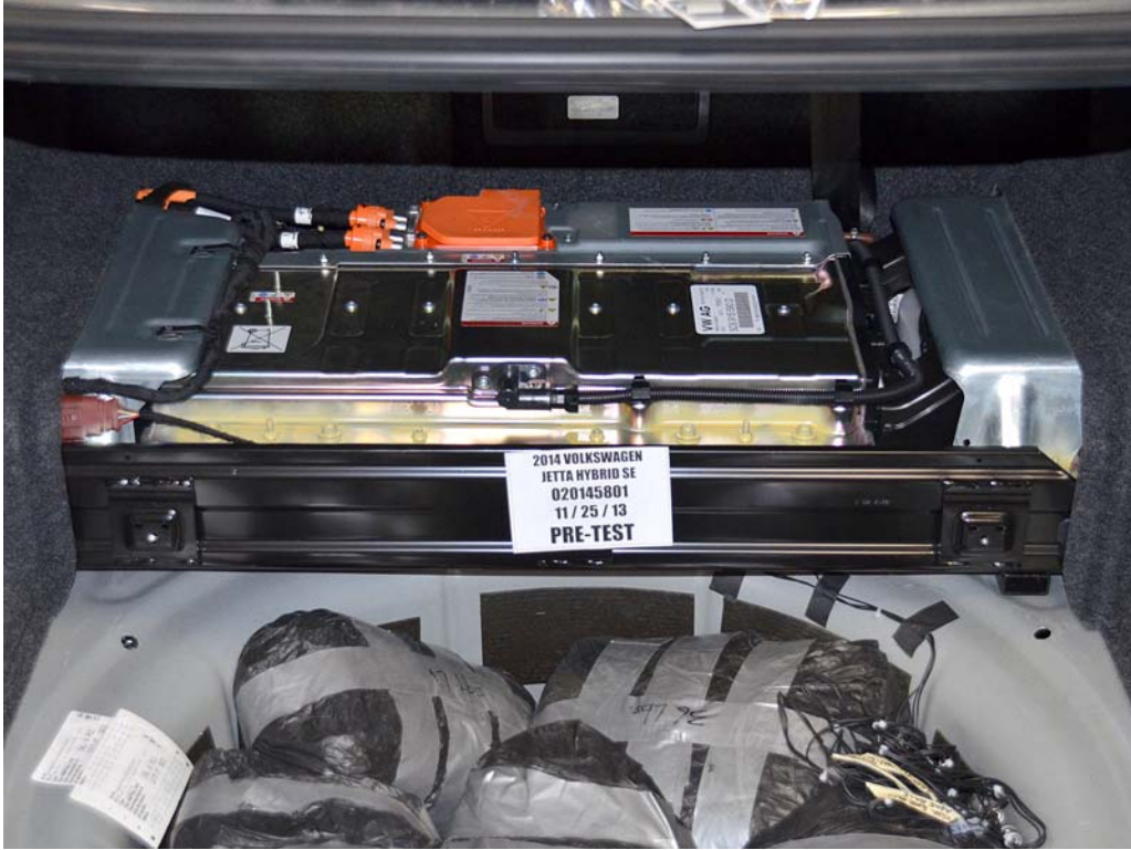
FIGURE 12a. Pre-Impact View of Propulsion Battery Box(s) or Container(s) which Holds Individual Battery Modules
