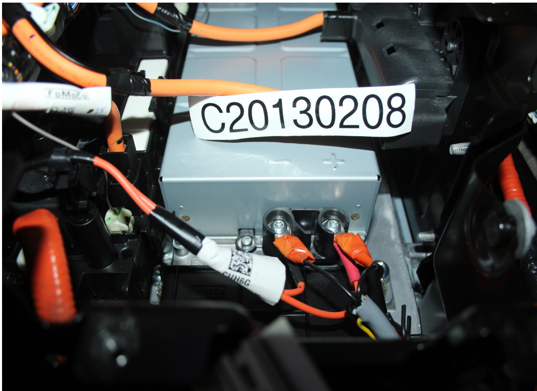
Post-Test Voltage Monitoring Leads Attached to Electric Energy Storage System
