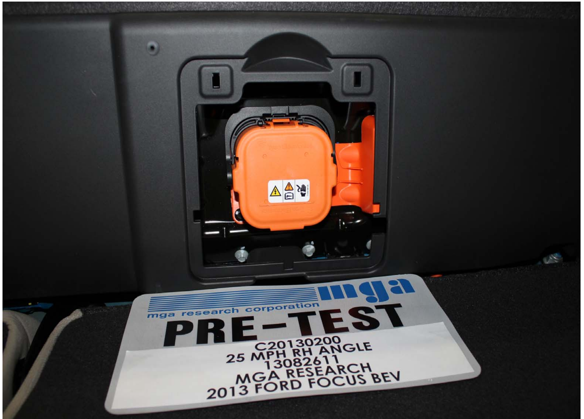
Pre-Test Manual High Voltage Service Disconnect in Place
