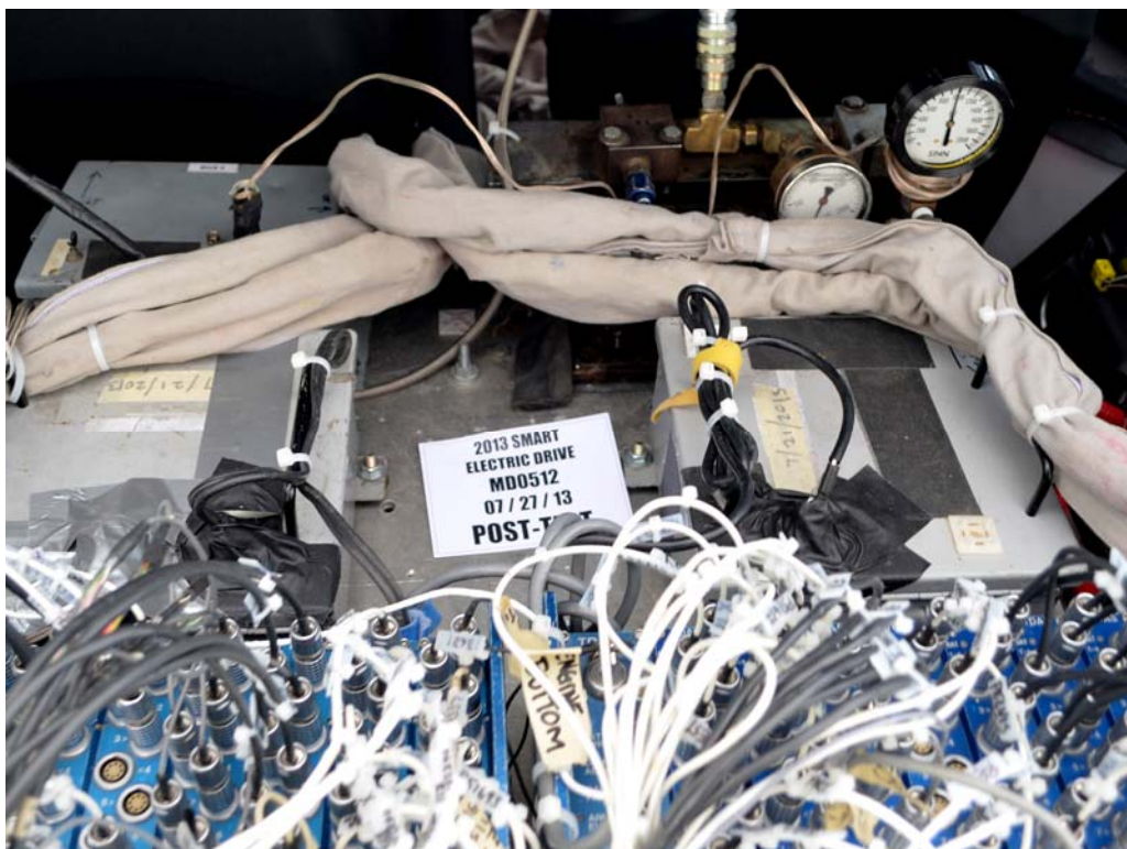
FIGURE 28. Post-Test Dummy Cable Routing
