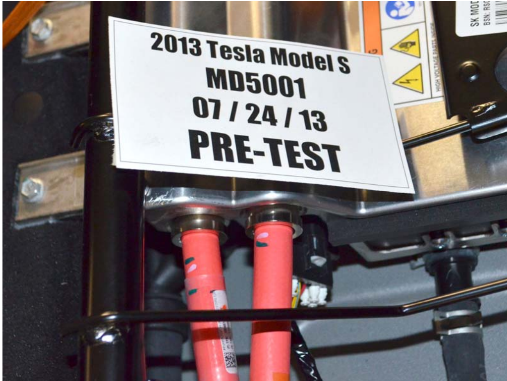
FIGURE 18d. Pre-Impact View of High Voltage Interconnect(s)
