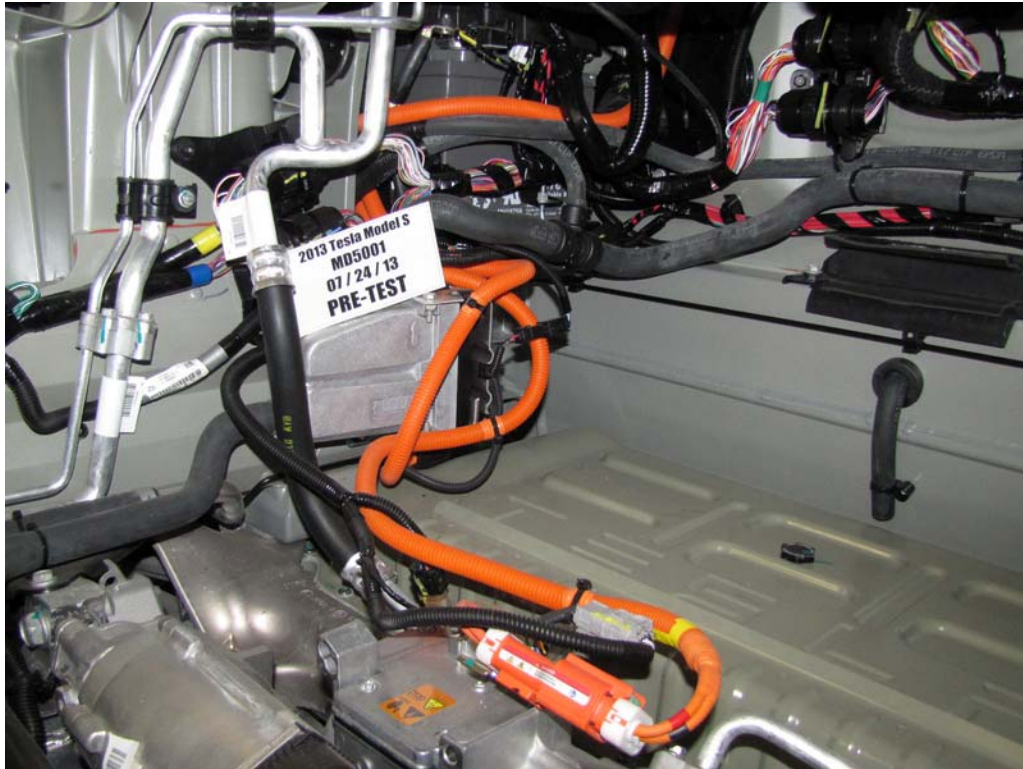
FIGURE 18. Pre-Impact View of High Voltage Interconnect(s)
