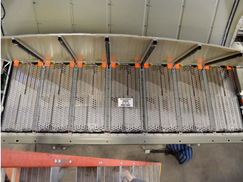
FIGURE 15a. Post-Impact View of Propulsion Battery Module(s)
