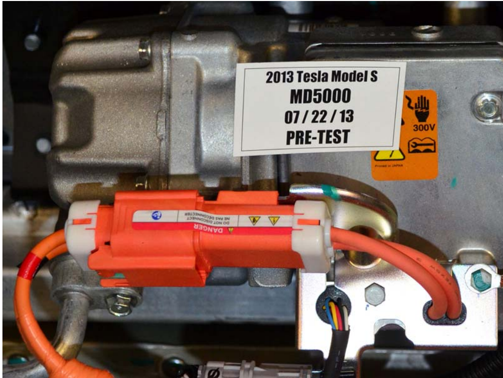
FIGURE 18a. Pre-Impact View of High Voltage Interconnect(s)
