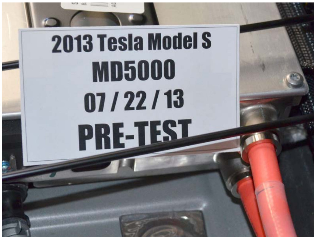
FIGURE 18f. Pre-Impact View of High Voltage Interconnect(s)
