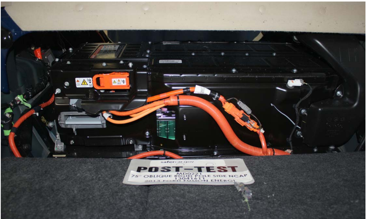
No. 010 Post-Impact Front View of Propulsion Battery
