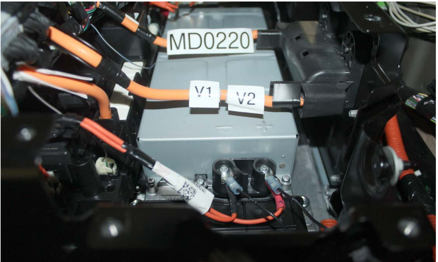
No. 022 Pre-Impact View of High Voltage Leads Attached
