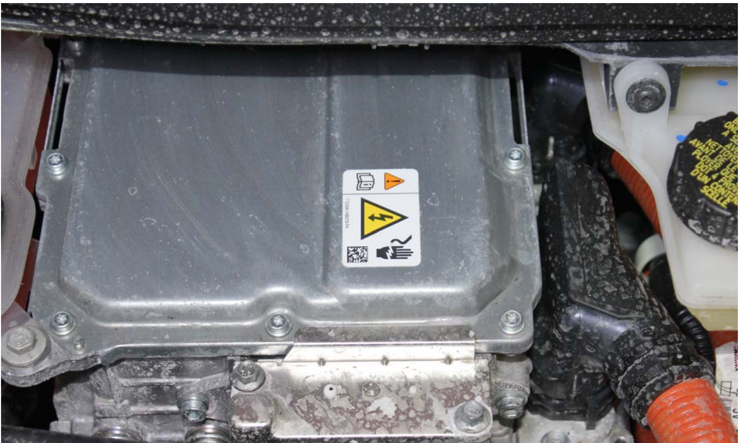
No. 002 Power Inverter Warning Label
