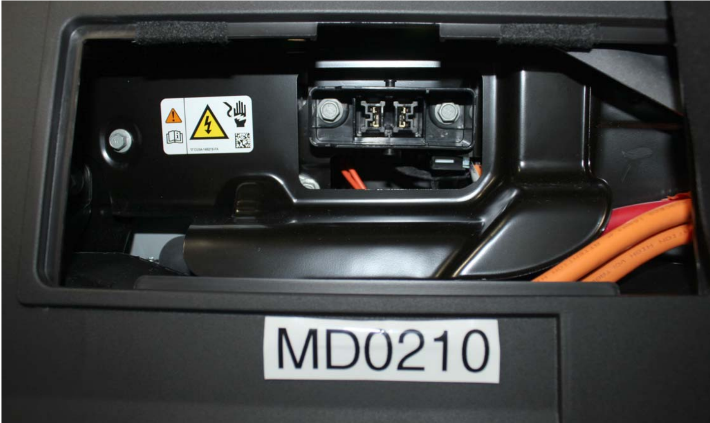
No. 007 Manual High Voltage Service Disconnect Removed
