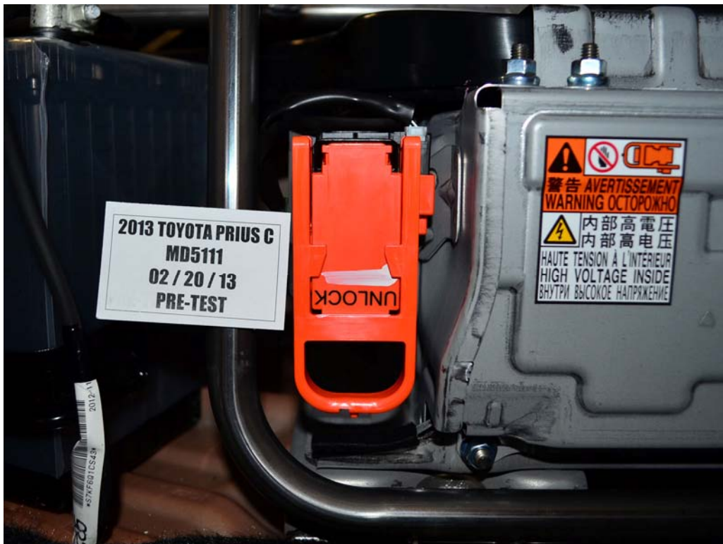
FIGURE 6. Manual High Voltage Service Disconnect In Place
