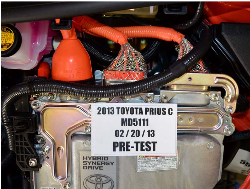
FIGURE 18. Pre-Impact View of High Voltage Interconnect
