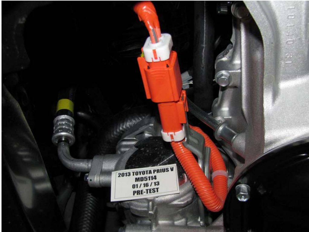
FIGURE 18. Pre-Impact View of High Voltage Interconnect(s)
