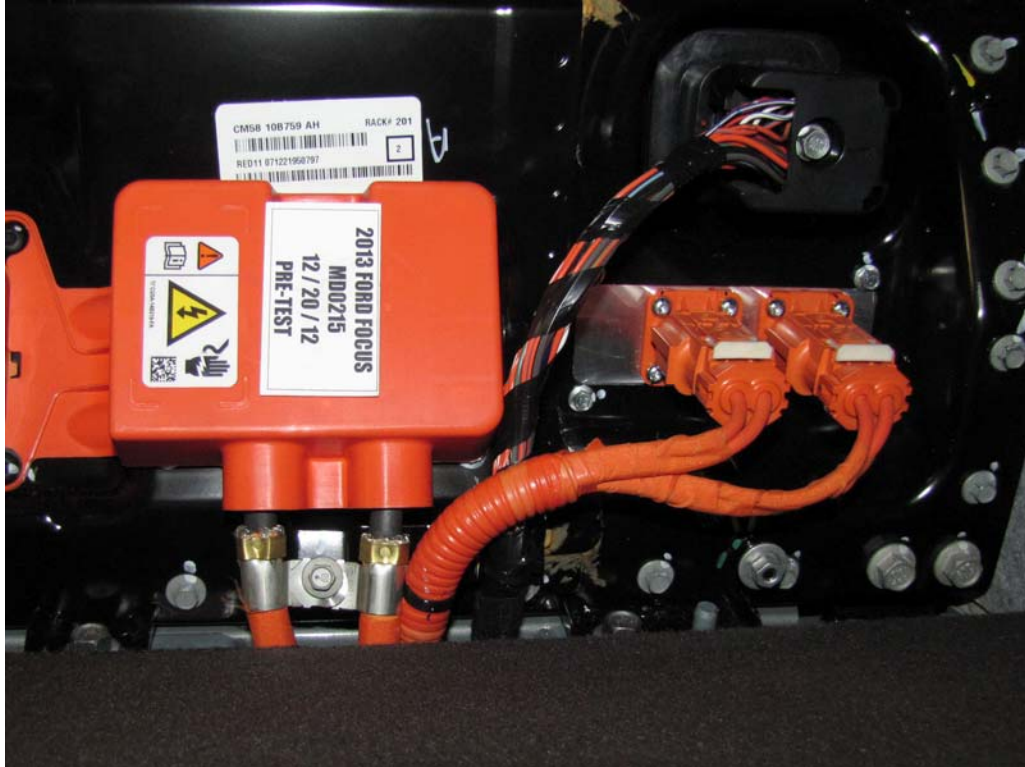
FIGURE 18a. Pre-Impact View of High Voltage Interconnect(s)
