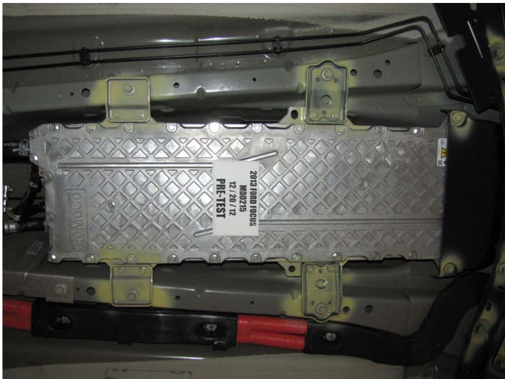
FIGURE 20. Pre-Impact View of Other Visible Electric Propulsion Components
