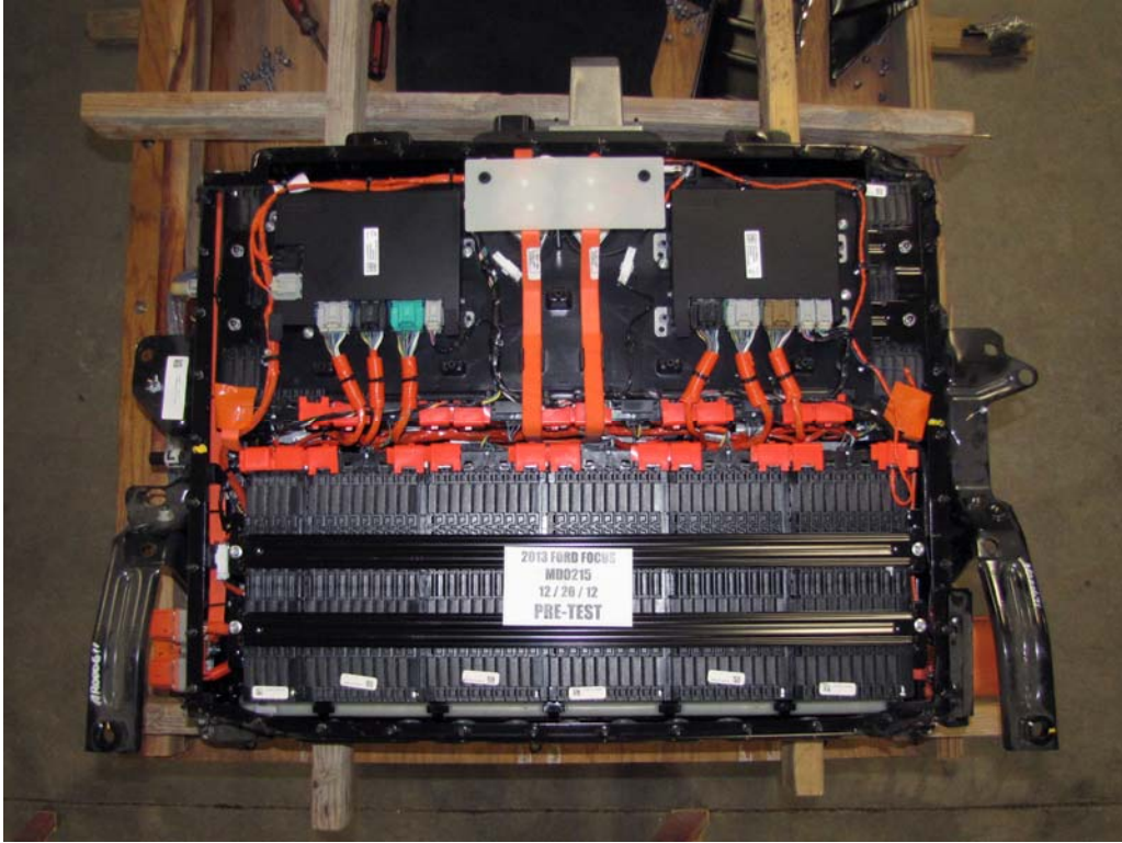
FIGURE 14a. Pre-Impact View of Battery Modules
