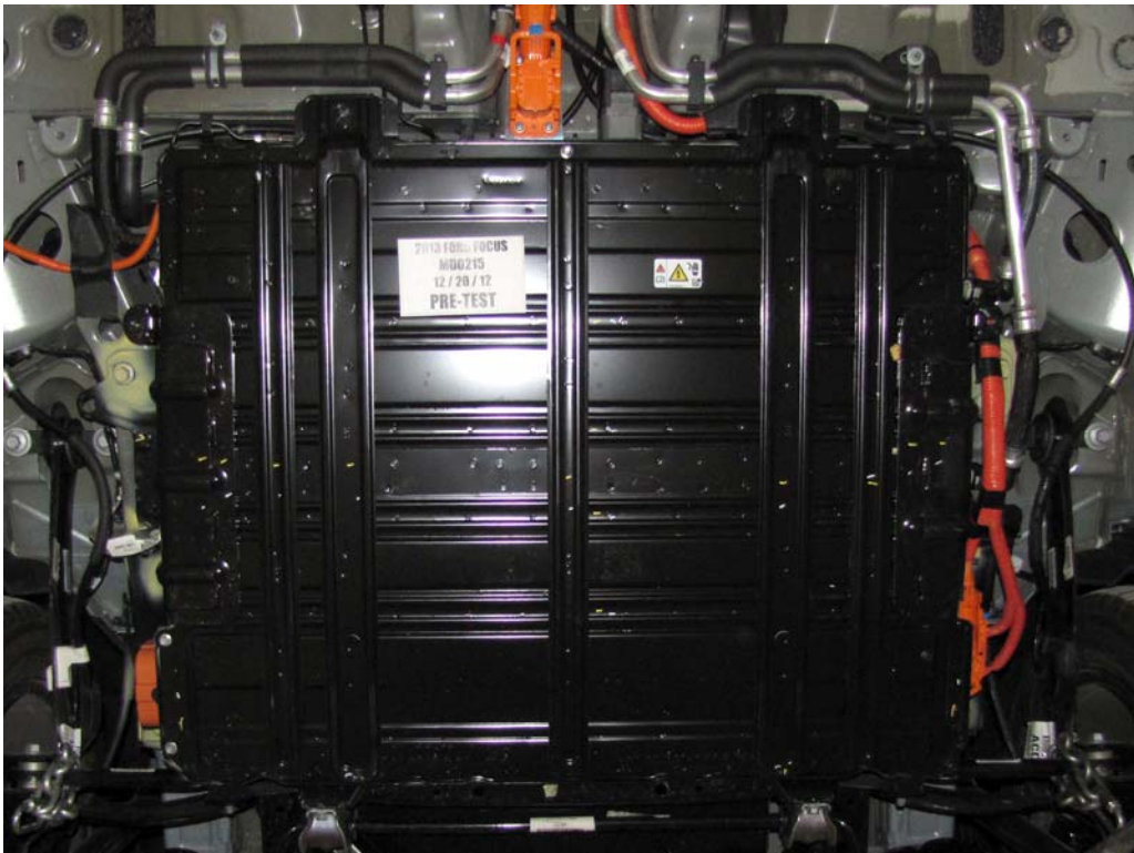
FIGURE 9b. Pre-Impact View of Propulsion Battery
