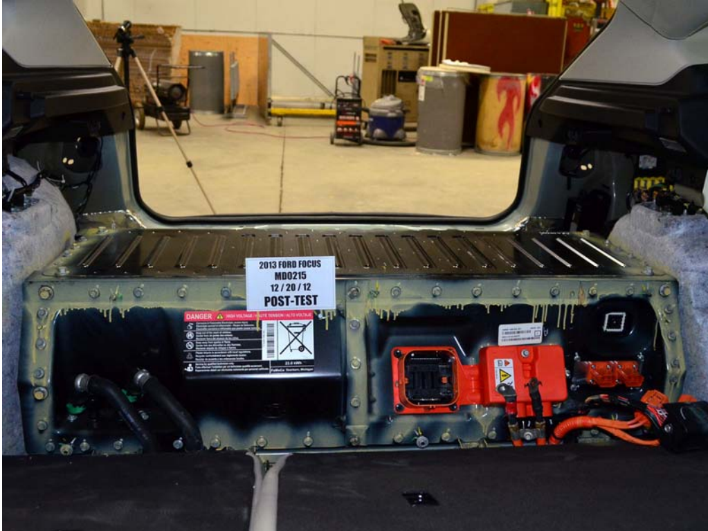
FIGURE 34. Post-Impact View of Vehicle Passenger Compartment Adjacent to Propulsion Battery
