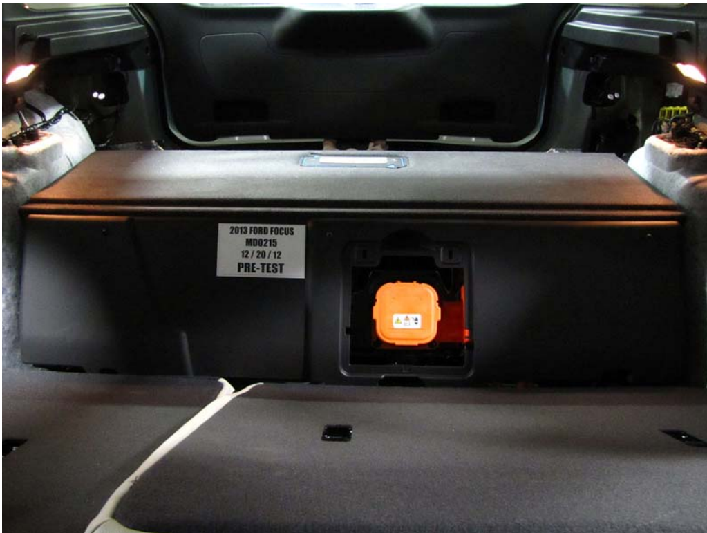
FIGURE 6. Manual High Voltage Service Disconnect In Place
