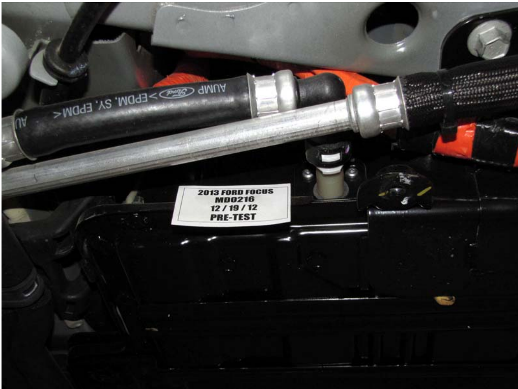
FIGURE 19. Pre-Impact View of Propulsion Battery Venting System(s)
