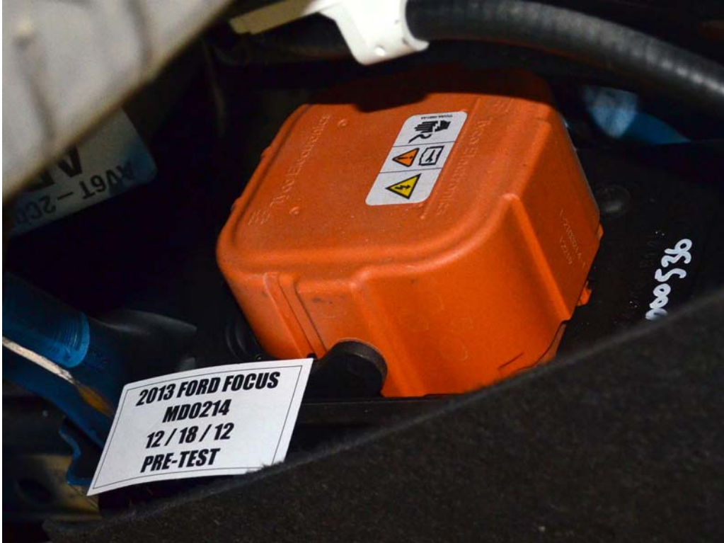
FIGURE 6a. Manual High Voltage Disconnect In Place
