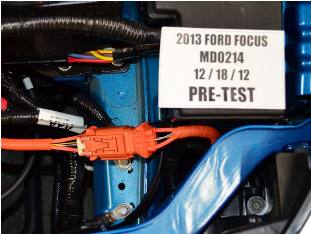
FIGURE 18. Pre-Impact View of High Voltage Interconnect(s)
