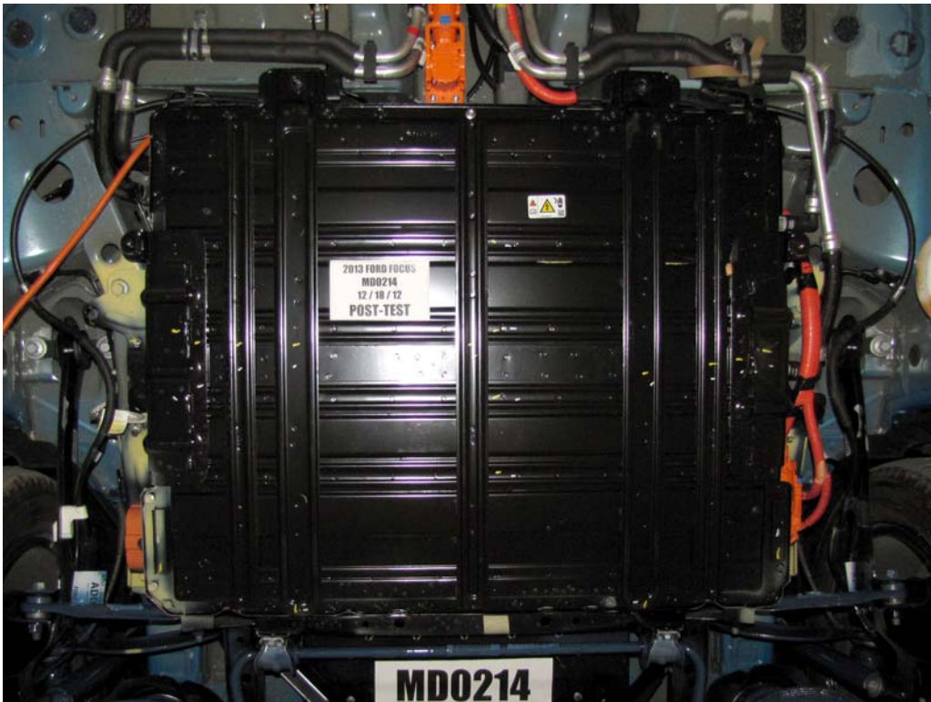
FIGURE 11. Post-Impact Rear View of Propulsion Battery
