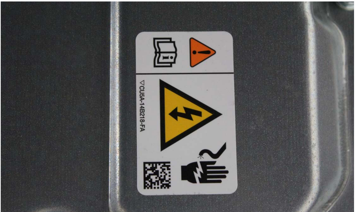
No. 002 Power Inverter Warning Label
