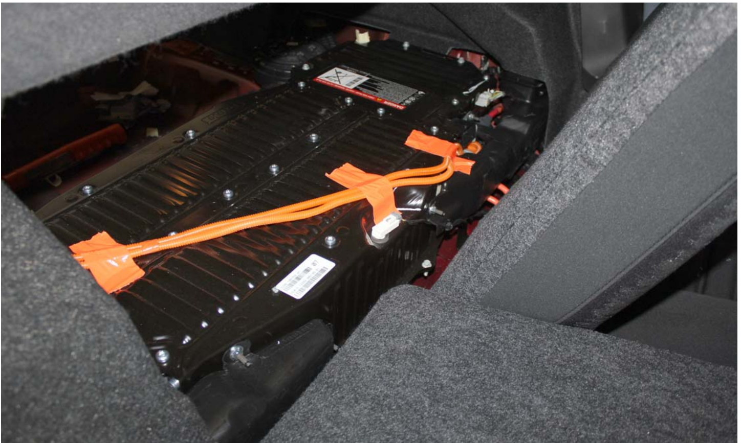
No. 010 Post-Impact Front View of Propulsion Battery
