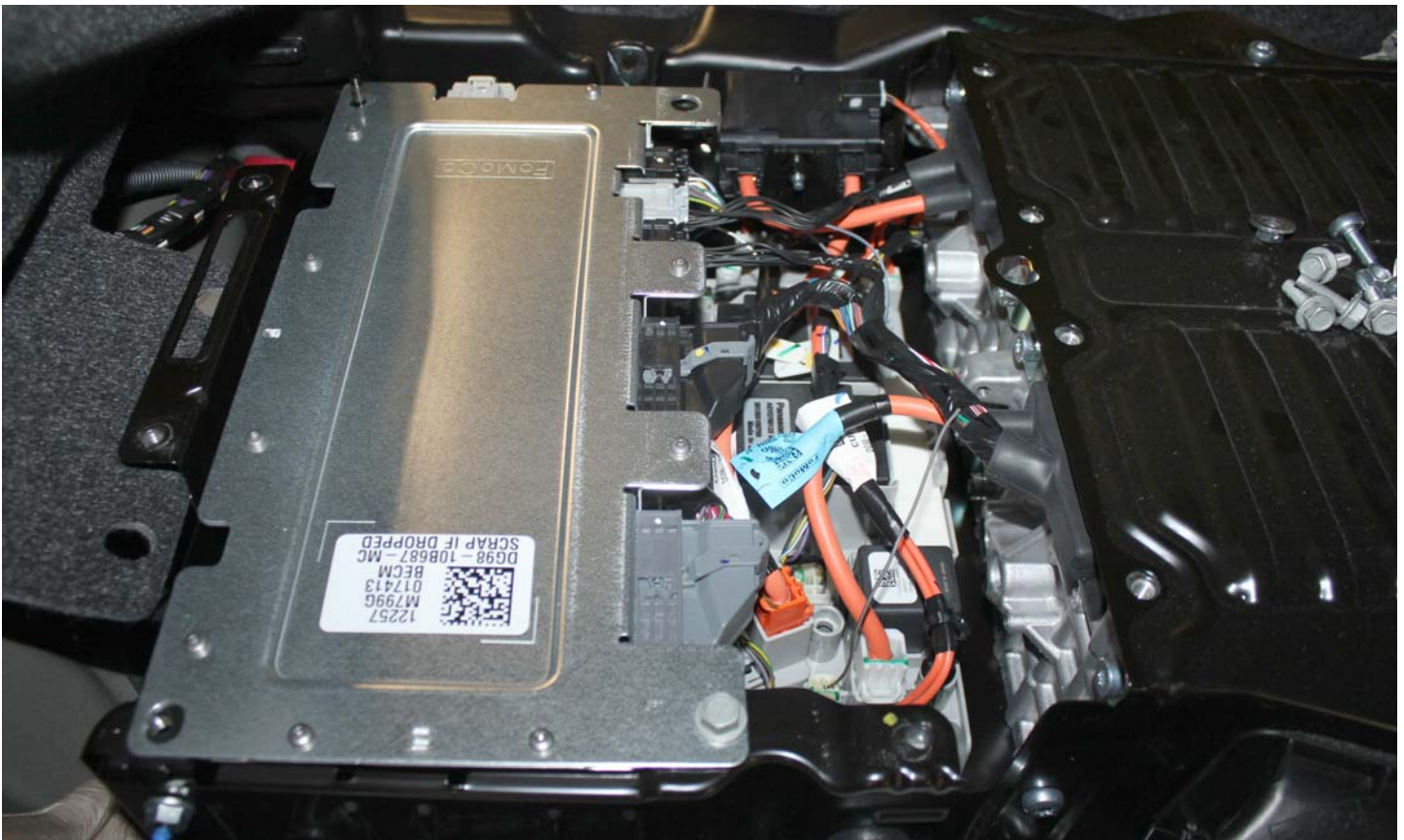
No. 018 Pre-Impact View of High Voltage Interconnect(s)
