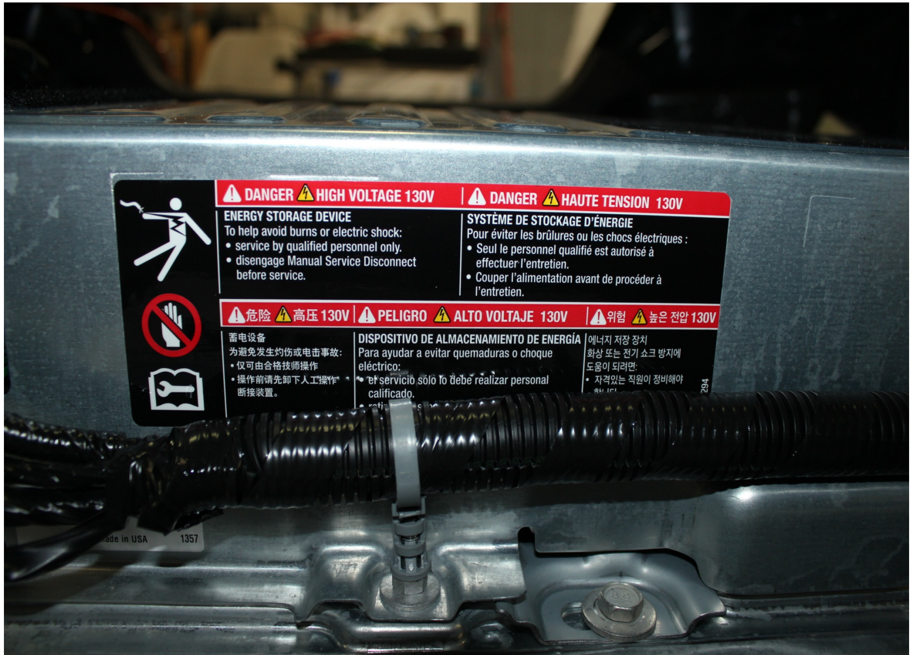
High Voltage Warning Label
