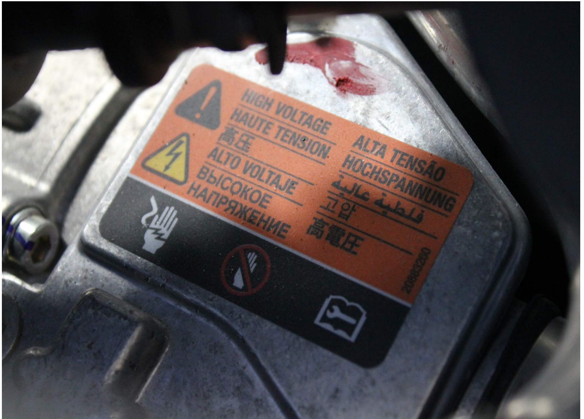
High Voltage Warning Label
