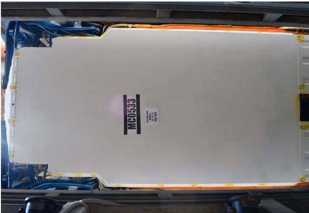
FIGURE 12. Pre-Impact View of Battery Box or Container Which Holds Individual Battery Modules
