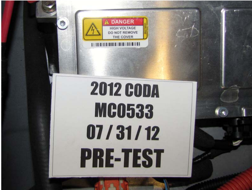
FIGURE 2a. Power Inverter Warning Label
