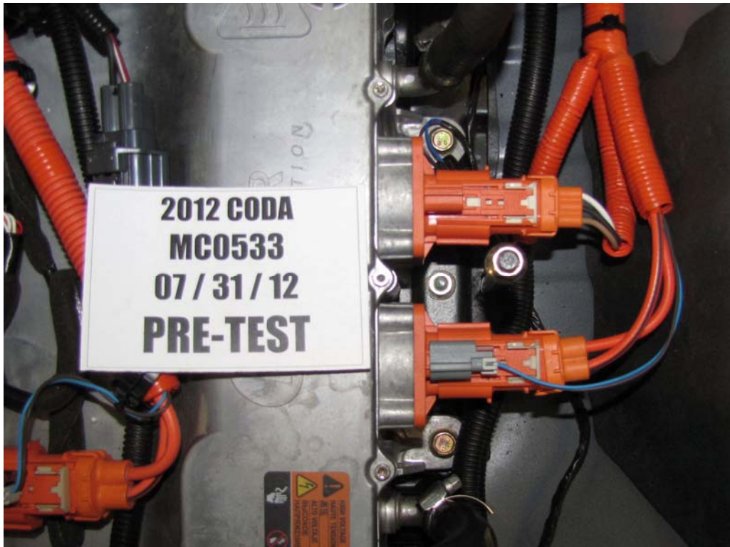
FIGURE 18b. Pre-Impact View of High Voltage Interconnect
