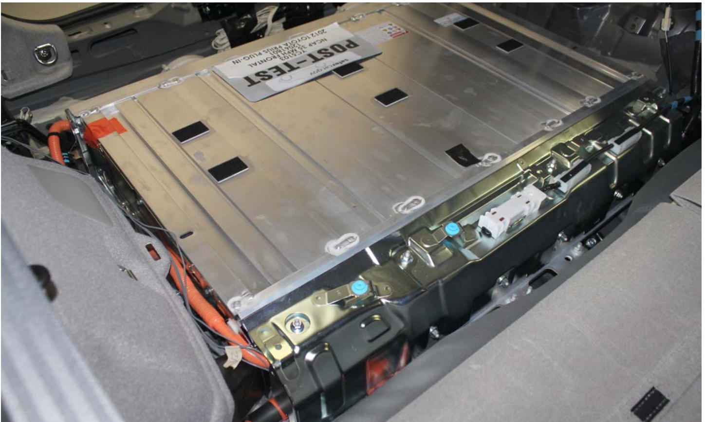
No. 011 Post-Impact Rear View of Propulsion Battery
