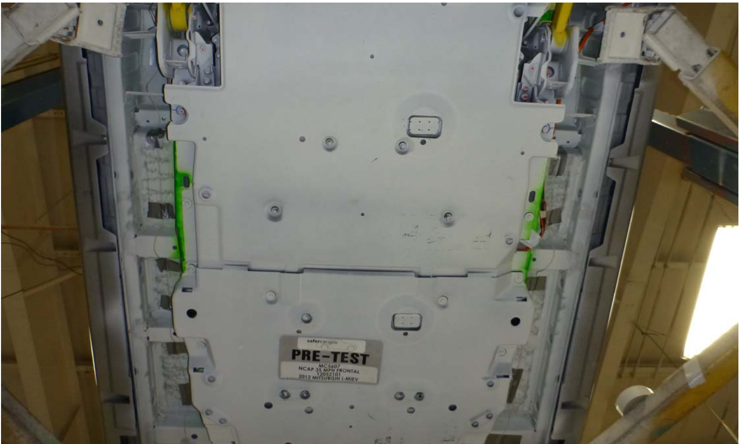
No. 012 Pre-Impact View of Battery Box(s) or Container(s) Which Holds Individual Battery Modules
