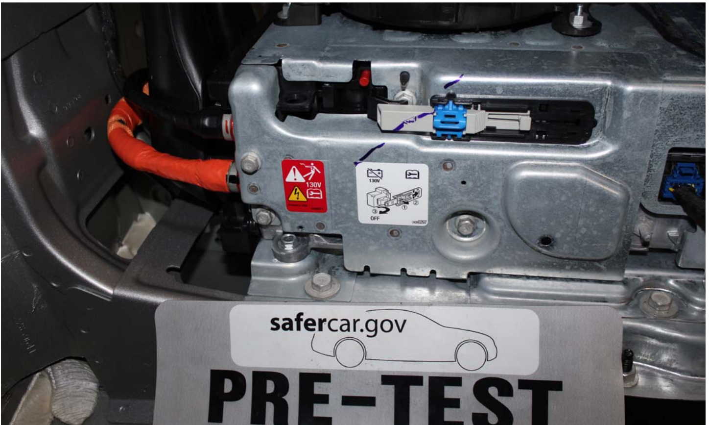
No. 006 Manual High Voltage Service Disconnect in Place
