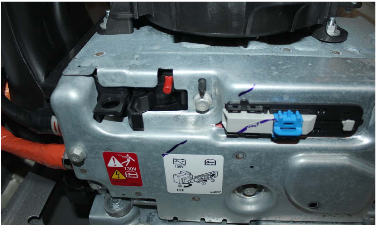
No. 007 Manual High Voltage Service Disconnect Removed
