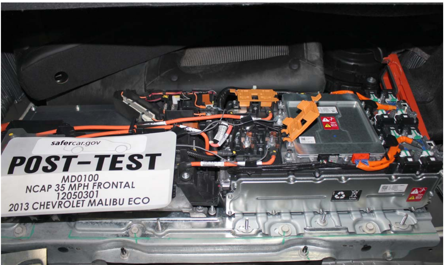
No. 015 Post-Impact View of Propulsion Battery Module(s)
