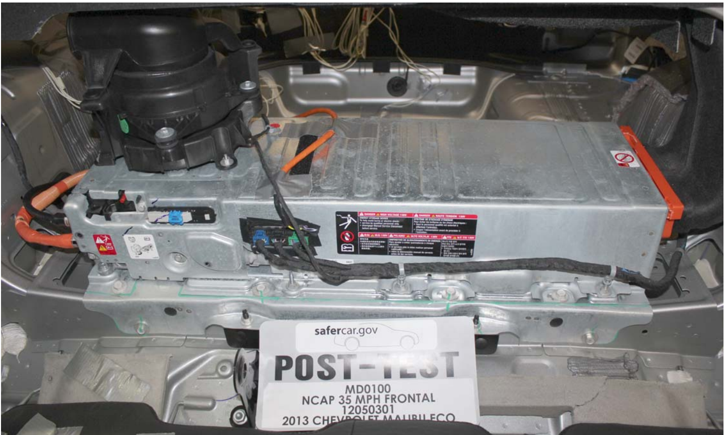
No. 010 Post-Impact Front View of Propulsion Battery
