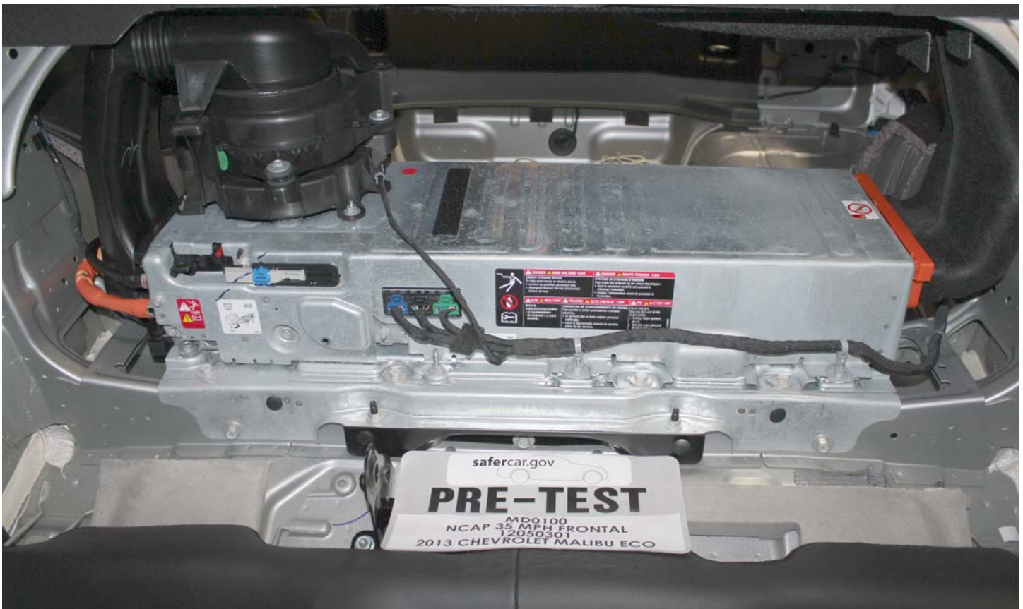
No. 019 Pre-Impact View Propulsion Battery Venting System(s)
