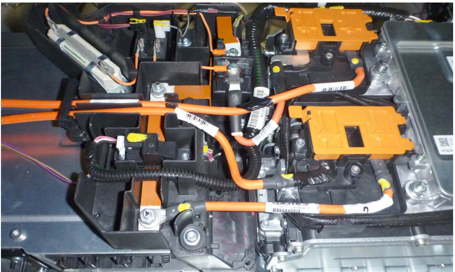
No. 015 Post-Impact View Of Propulsion Battery Module(S)
