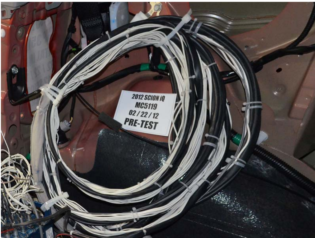
FIGURE 27. Pre-Test Dummy Cable Routing
