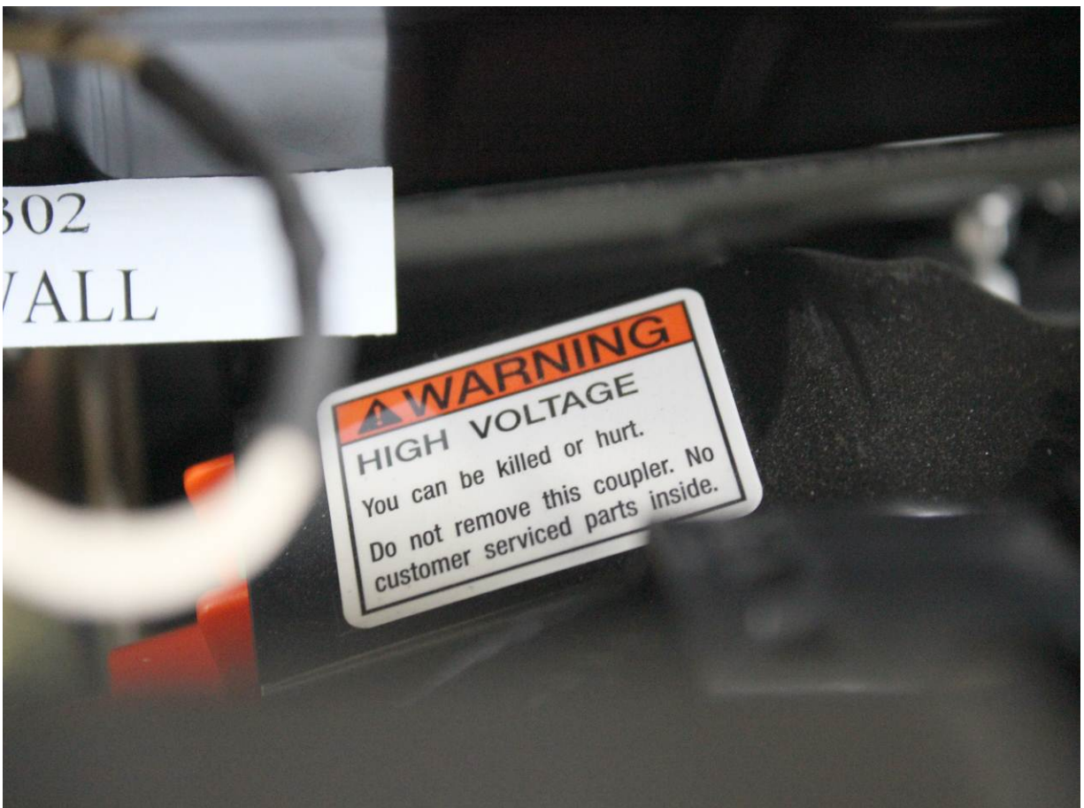
High Voltage Warning Label
