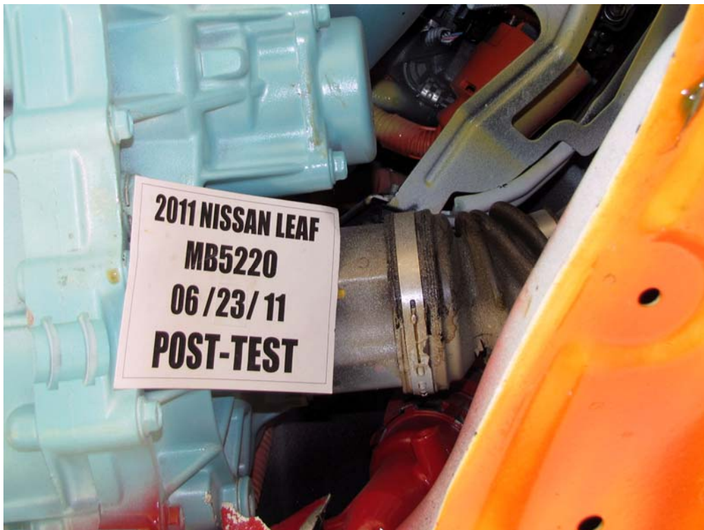
FIGURE 99. Post-Test High Voltage Connections
