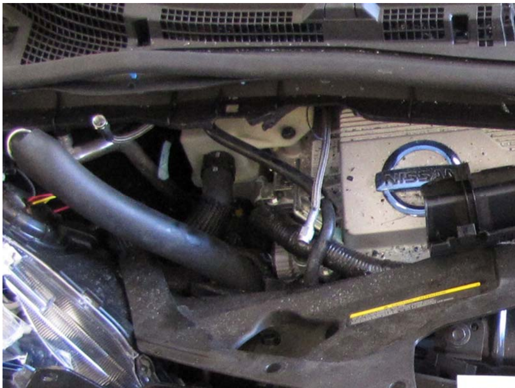
FIGURE 97. Post-Test High Voltage Connections
