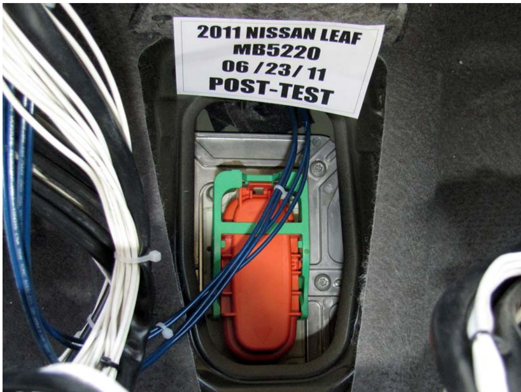
FIGURE 79. Post-Test Propulsion Battery Disconnect
