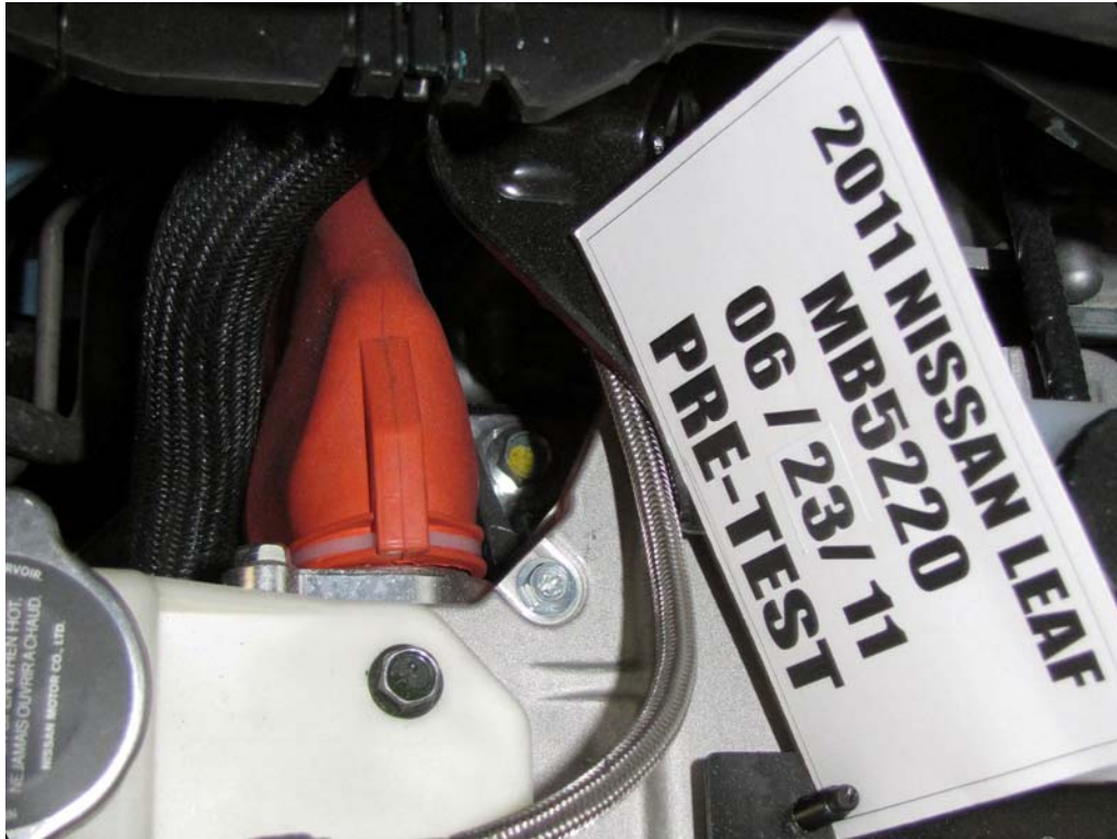
FIGURE 96. Pre-Test High Voltage Connections
