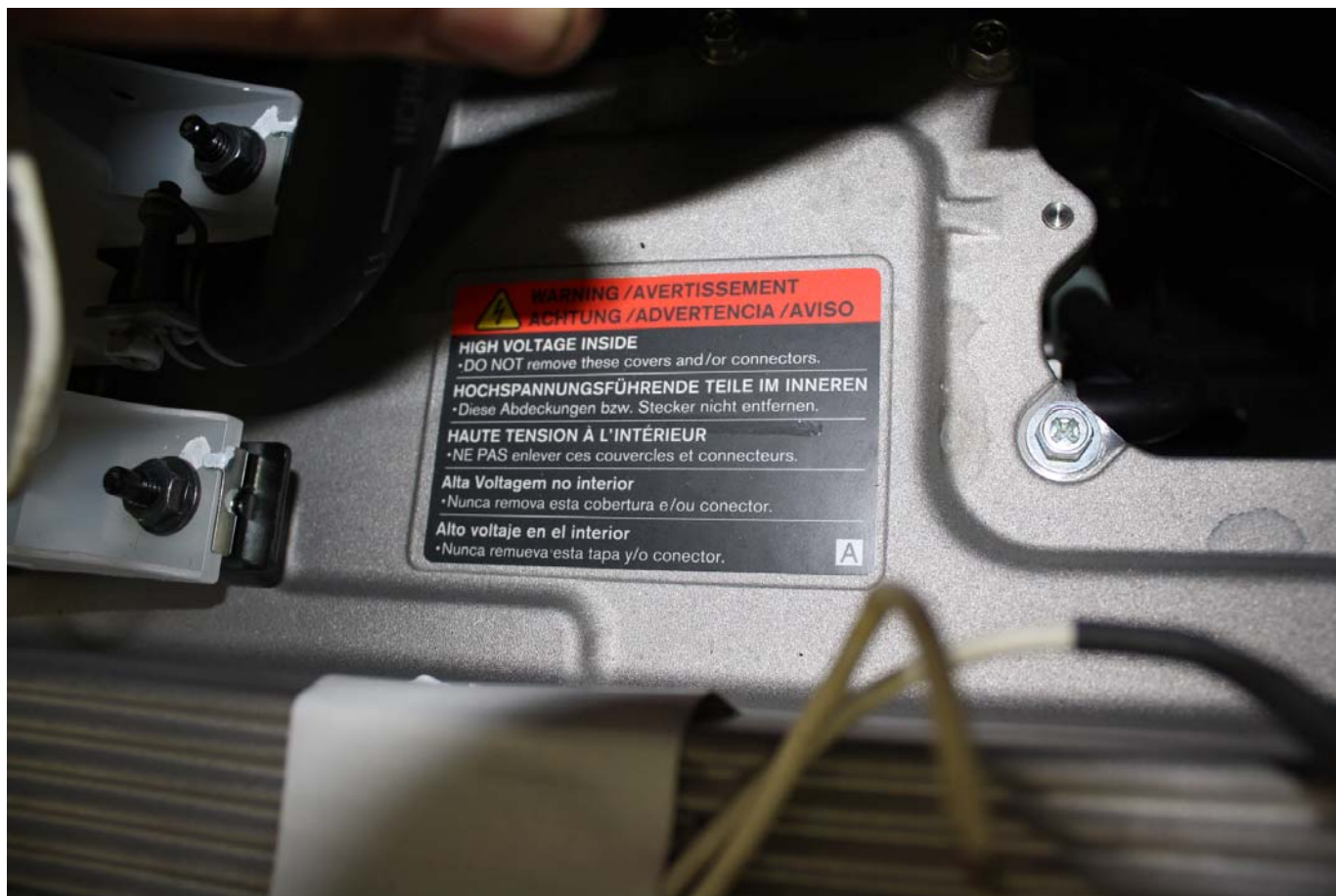
Power Inverter Warning Label
