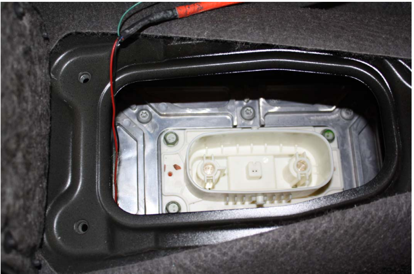
Manual High Voltage Service Disconnect
