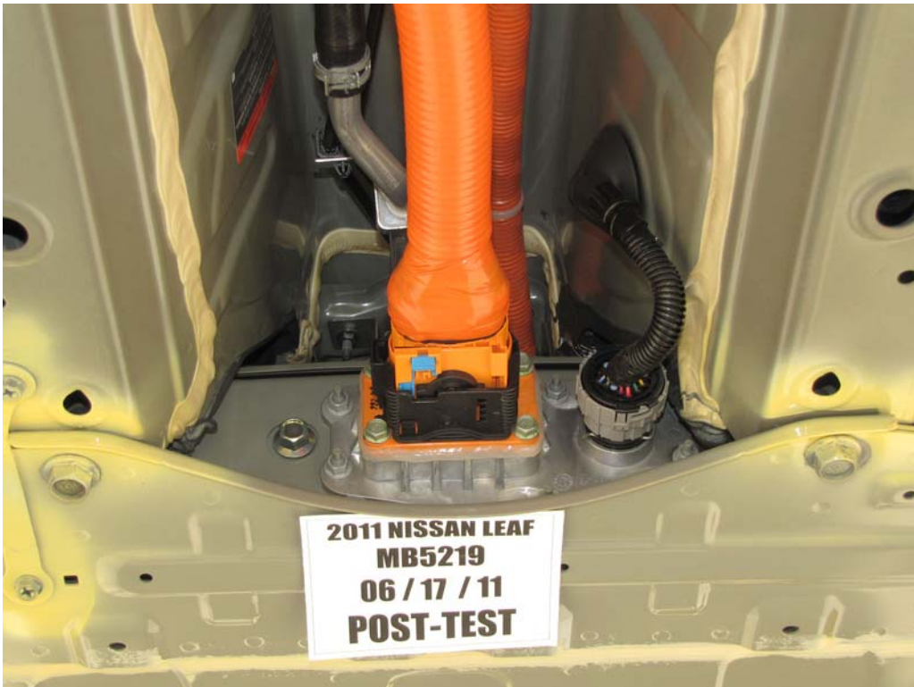
FIGURE 134. Post-Test High Voltage Connections
