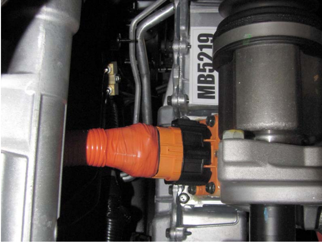
FIGURE 131. Pre-Test High Voltage Connections
