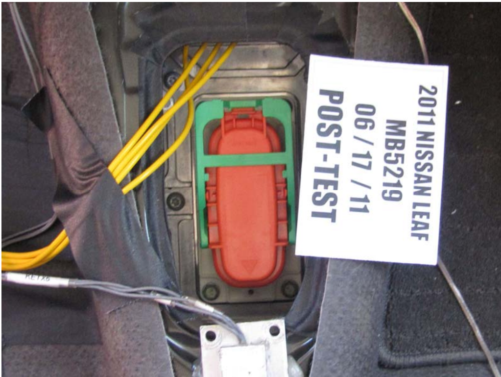
FIGURE 110. Post-Test Propulsion Battery Disconnect
