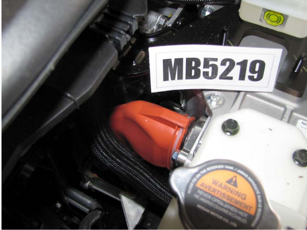
FIGURE 127. Pre-Test High Voltage Connections
