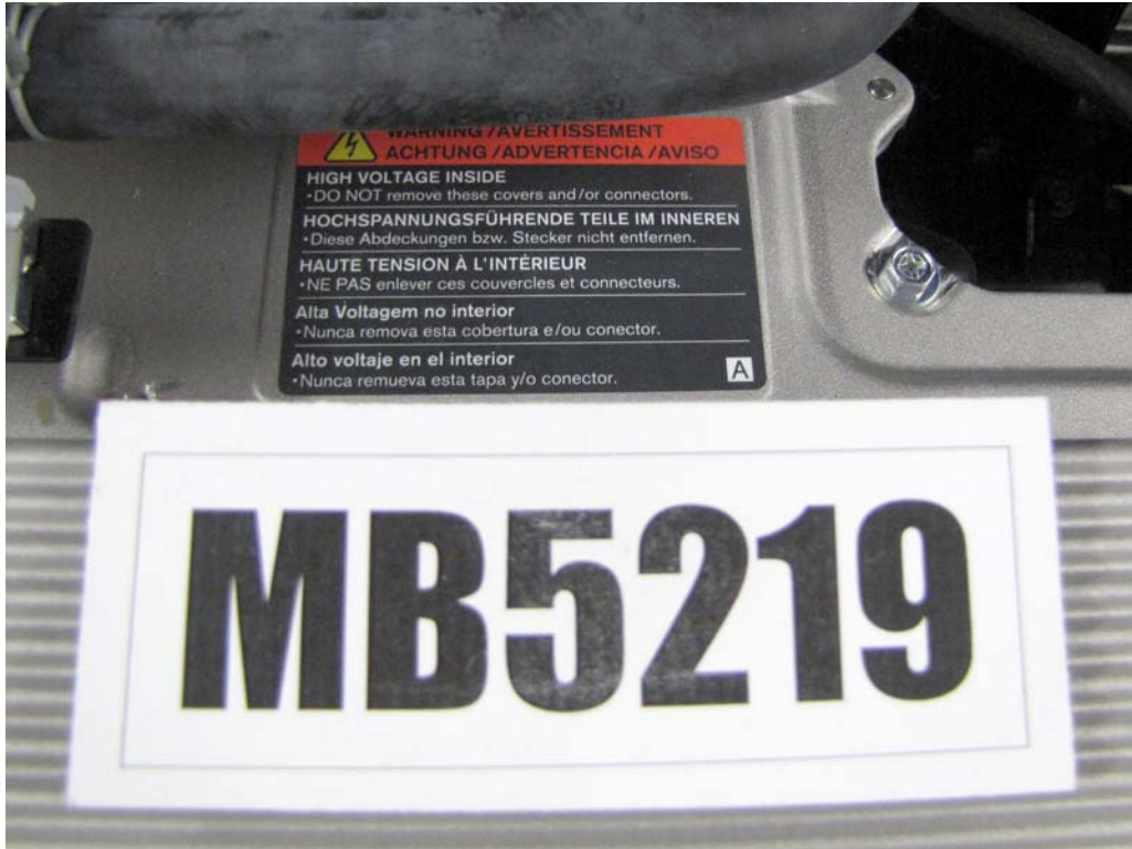
FIGURE 105. Electric System Label
