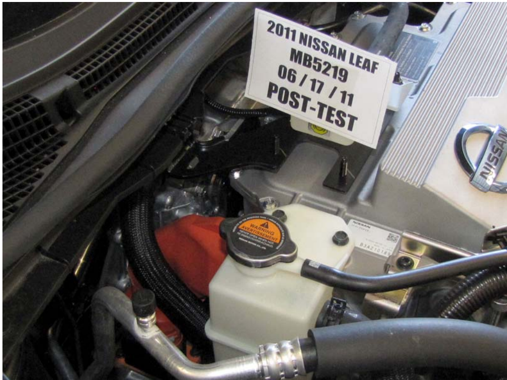
FIGURE 128. Post-Test High Voltage Connections
