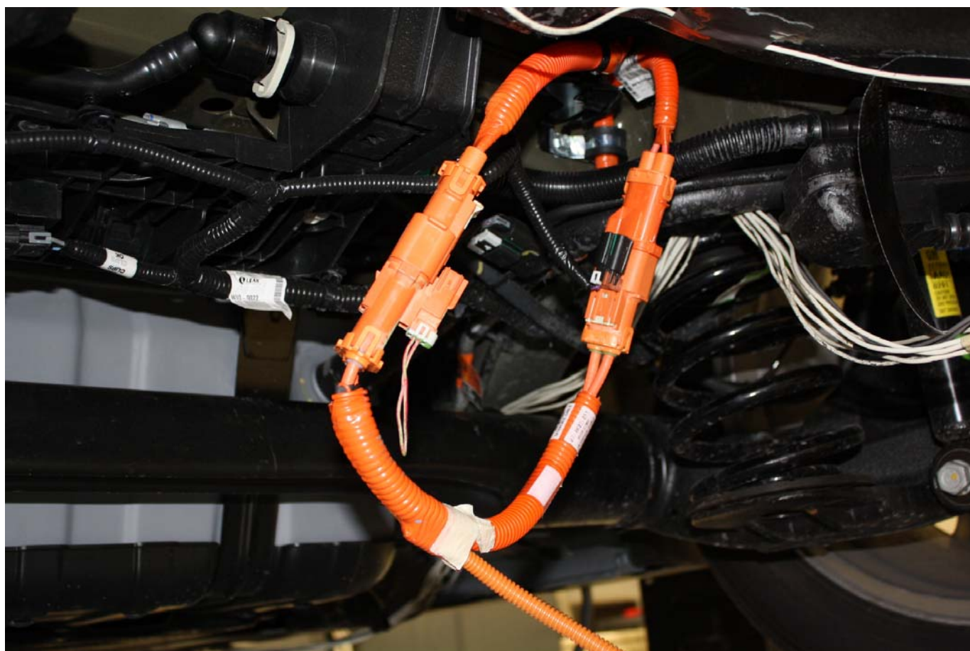
Close-Up of High Voltage Leads Attached
