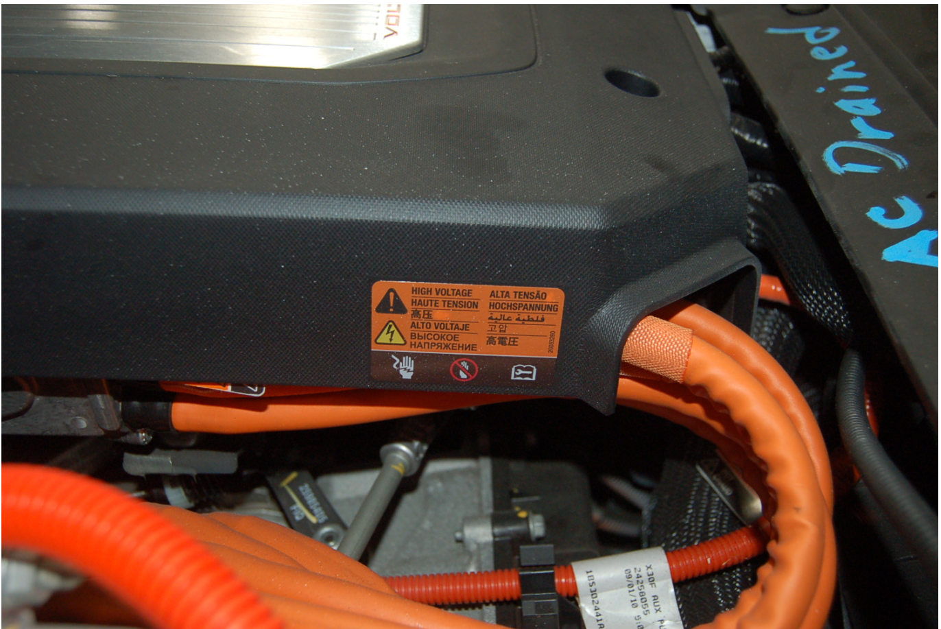
Power Inverter Warning Label
