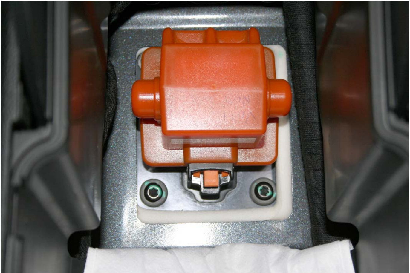
Manual High Voltage Service Disconnect
