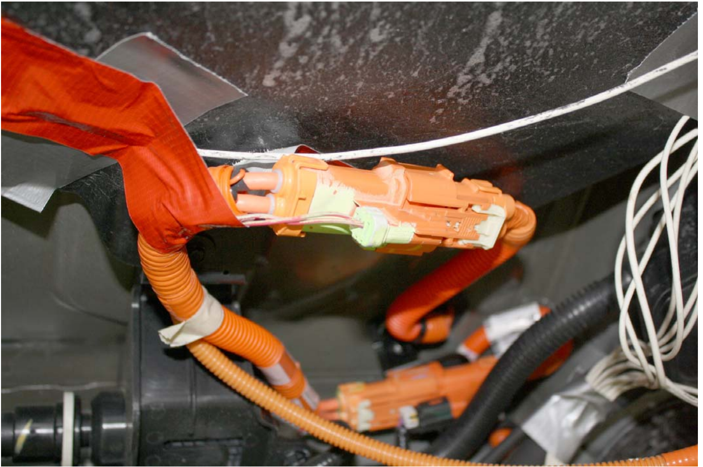
Close-Up of High Voltage Leads Attached
