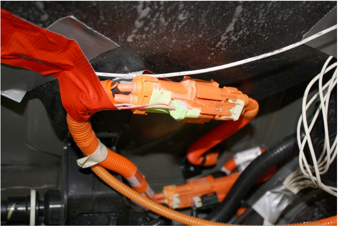
Close-Up of High Voltage Leads Attached
