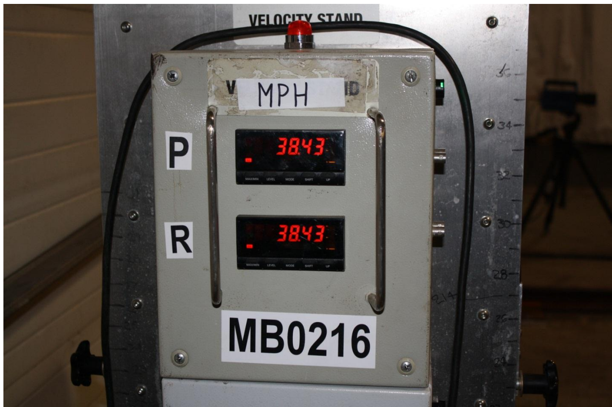
Figure A-92: Post-Test Primary and Redundant Speed Trap Read-Out
