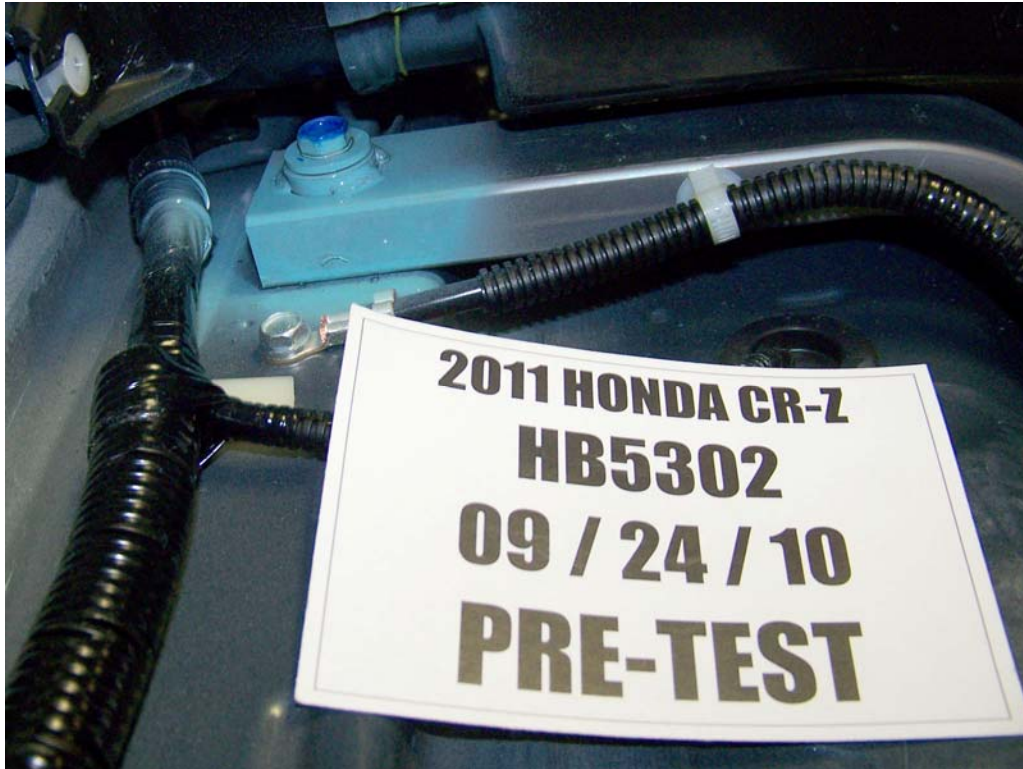
FIGURE 93. Pre-Test Battery Mounting Hardware
