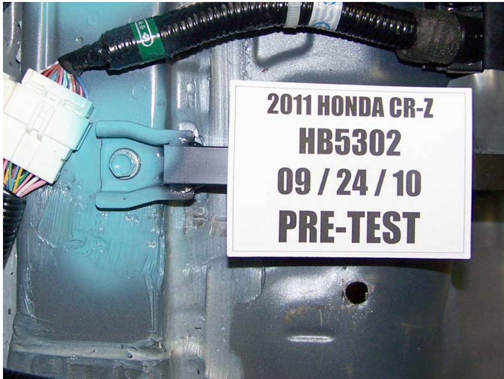
FIGURE 89. Pre-Test Battery Mounting Hardware
