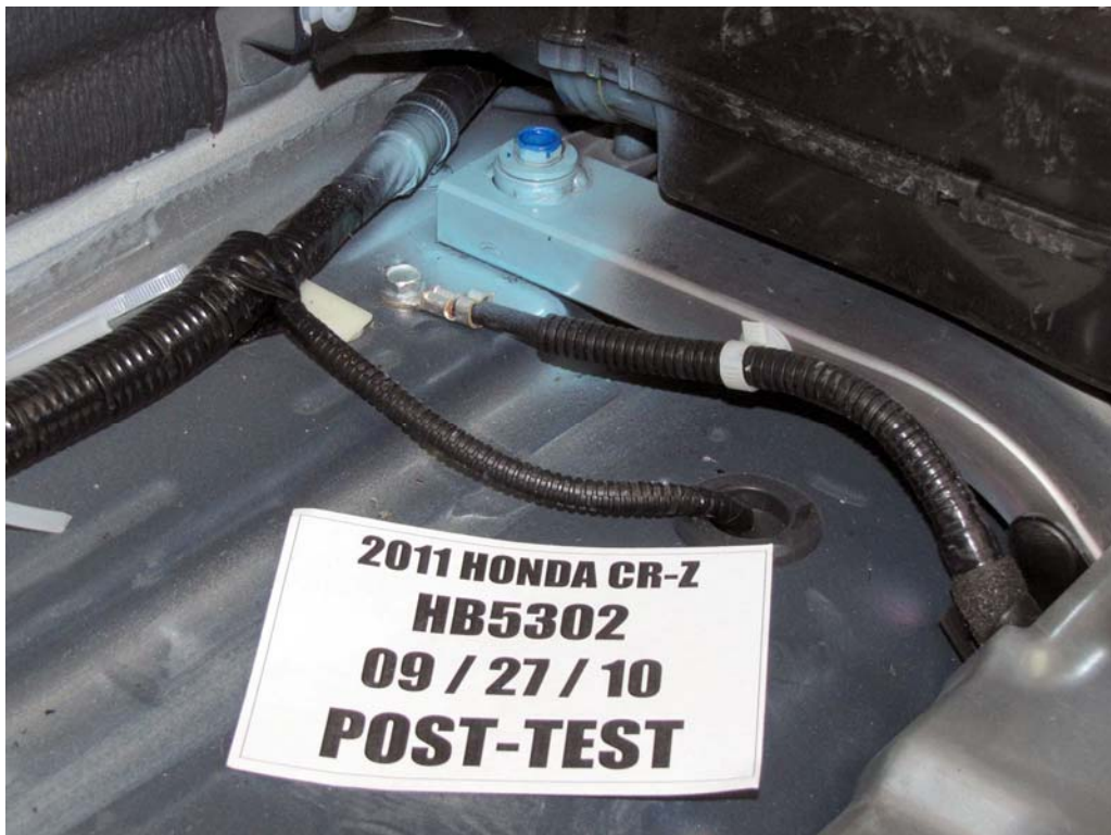
FIGURE 94. Post-Test Battery Mounting Hardware
