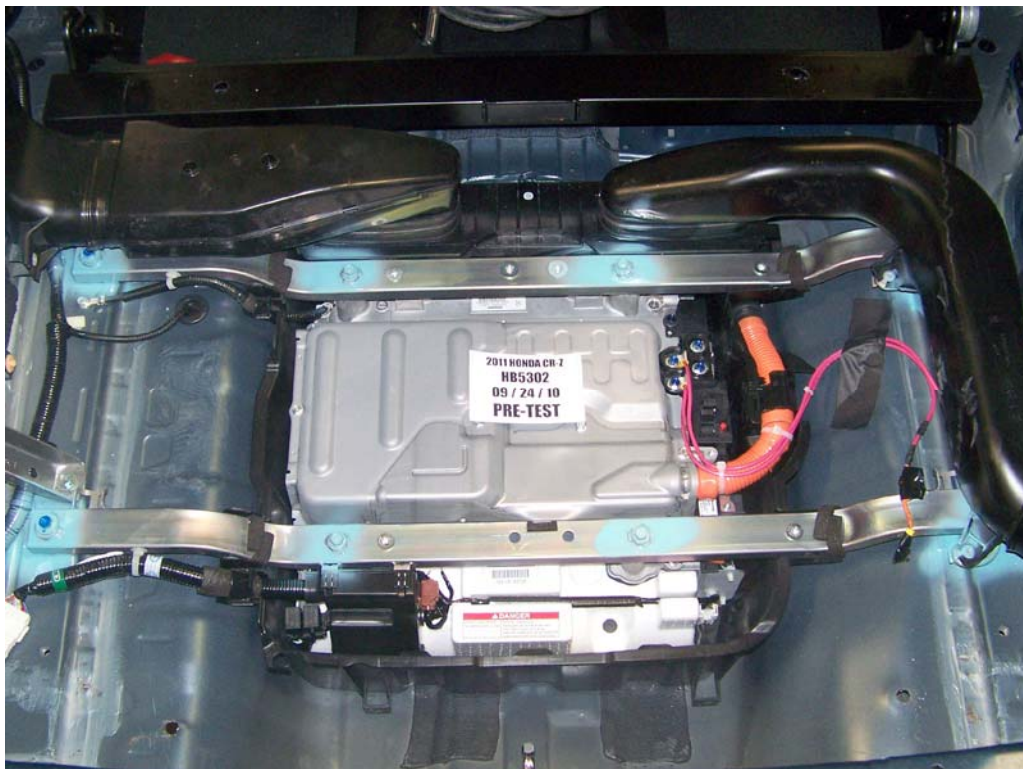
FIGURE 80. Pre-Test Battery Compartment
