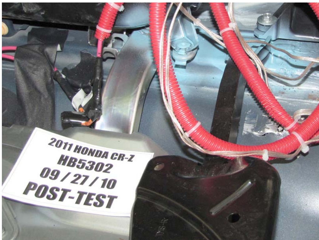
FIGURE 92. Post-Test Battery Mounting Hardware
