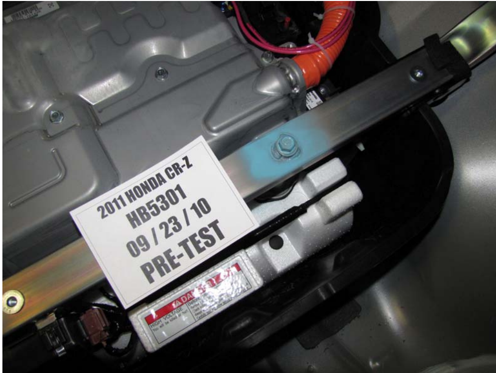
FIGURE 138. Pre-Test Battery Mounting Hardware
