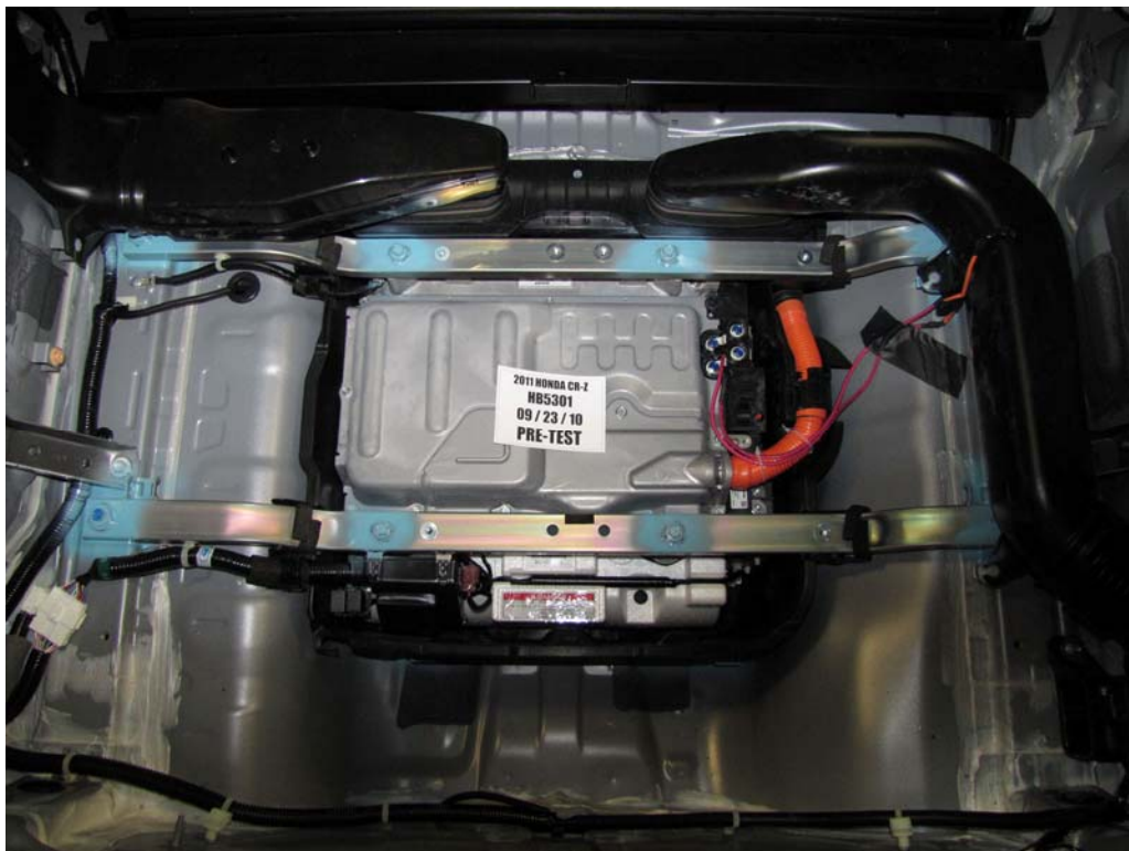
FIGURE 111. Pre-Test Battery Compartment
