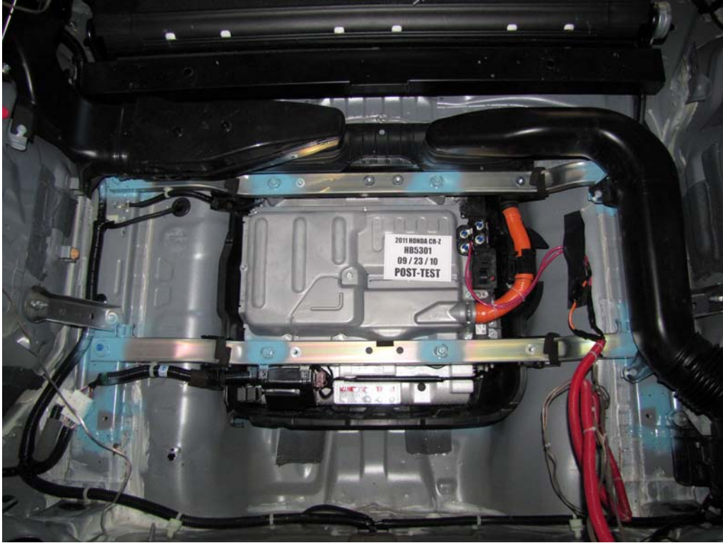
FIGURE 112. Post-Test Battery Compartment
