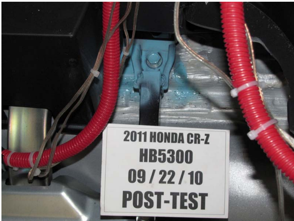
FIGURE 90. Post-Test Battery Mounting Hardware
