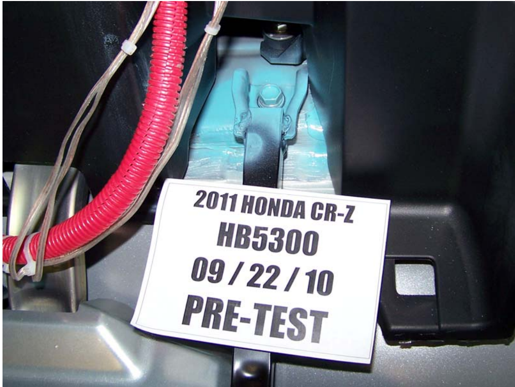
FIGURE 89. Pre-Test Battery Mounting Hardware
