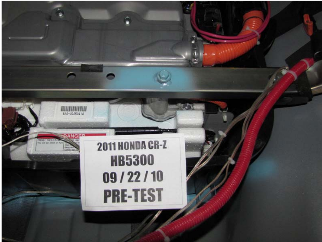
FIGURE 105. Pre-Test Battery Mounting Hardware
