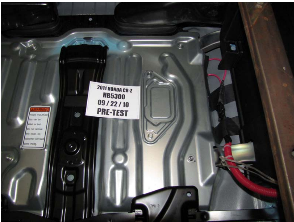
FIGURE 80. Pre-Test Propulsion Battery Disconnect
