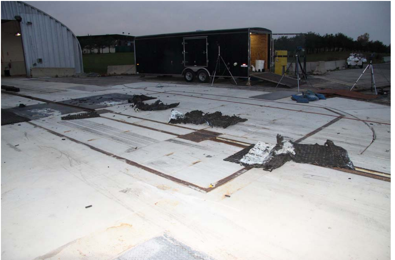
Figure A-64 Post-Test Mat Displacement – View 1
