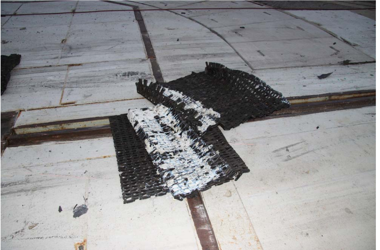
Figure A-70 Post-Test Mat Displacement – View 7
