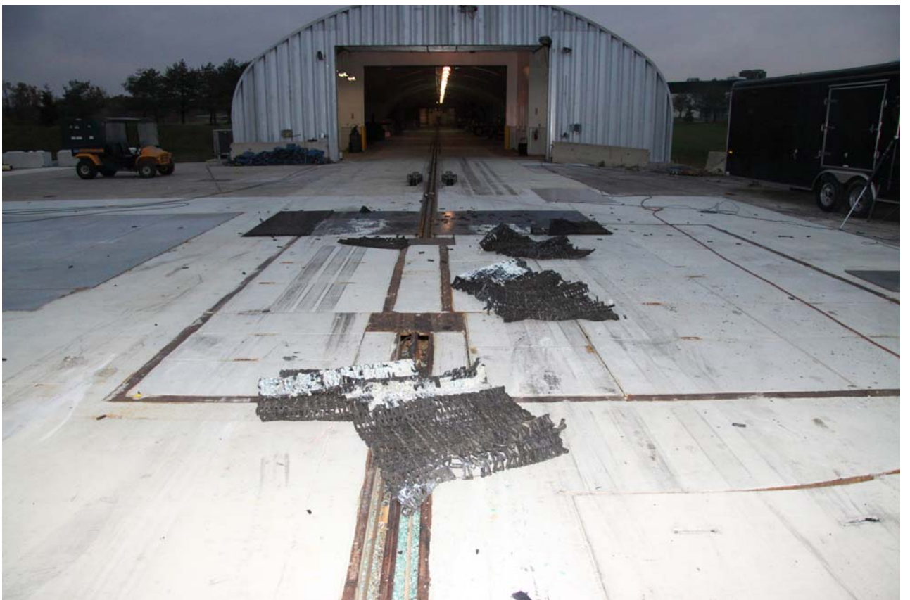
Figure A-65 Post-Test Mat Displacement – View 2
