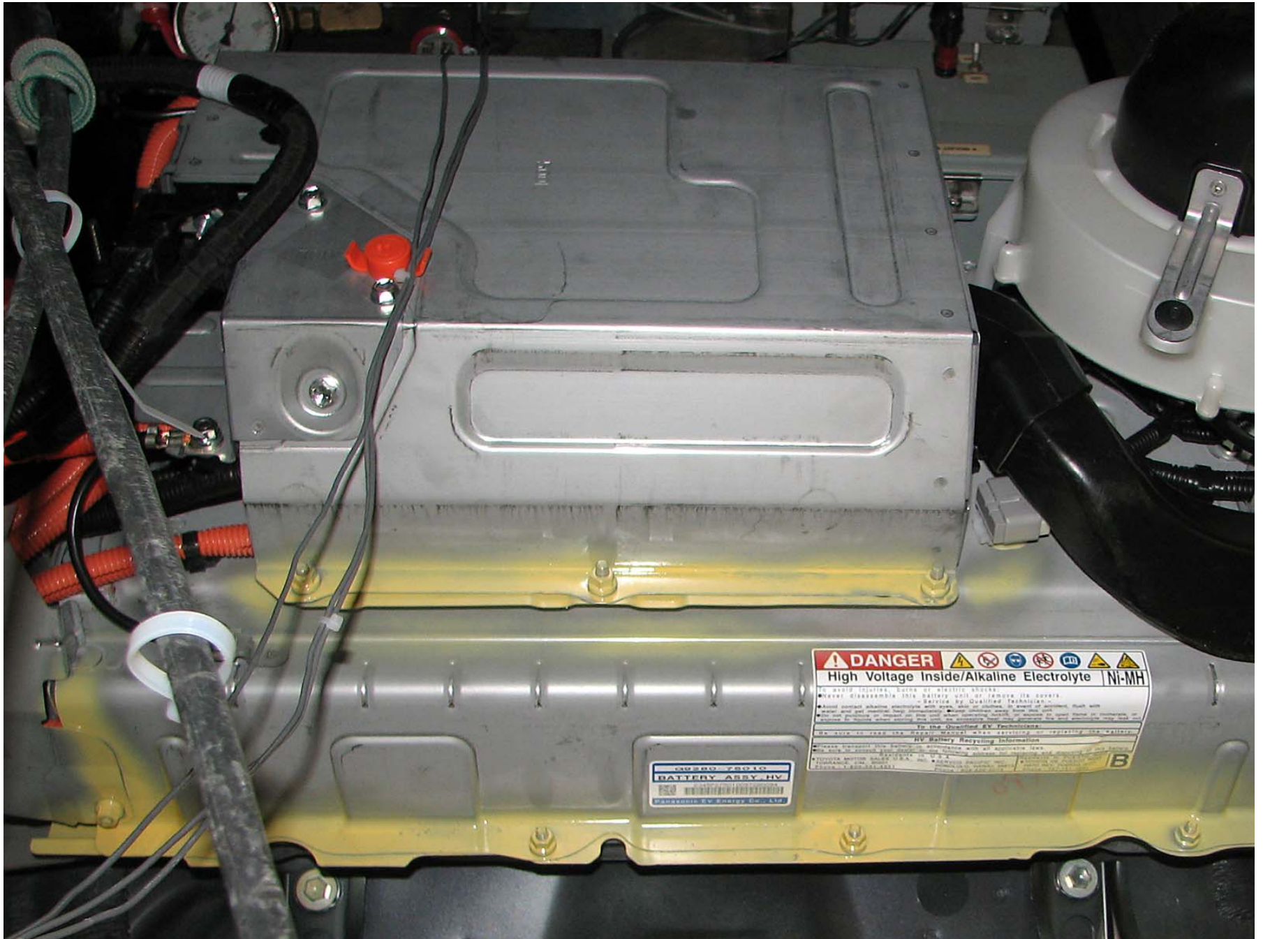
Figure A-69: Pre-Test View of Battery Compartment
