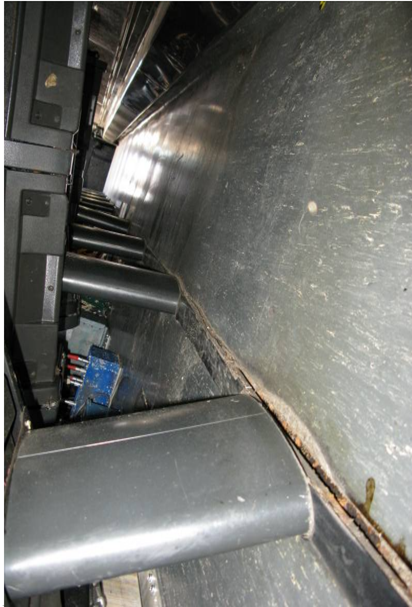
Post-Test Interior Damage View 11
