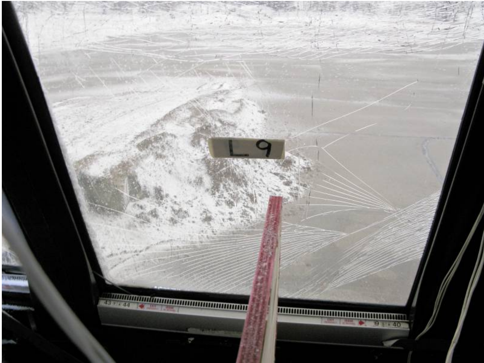
Post-Test Left Side Window 9 Interior View
