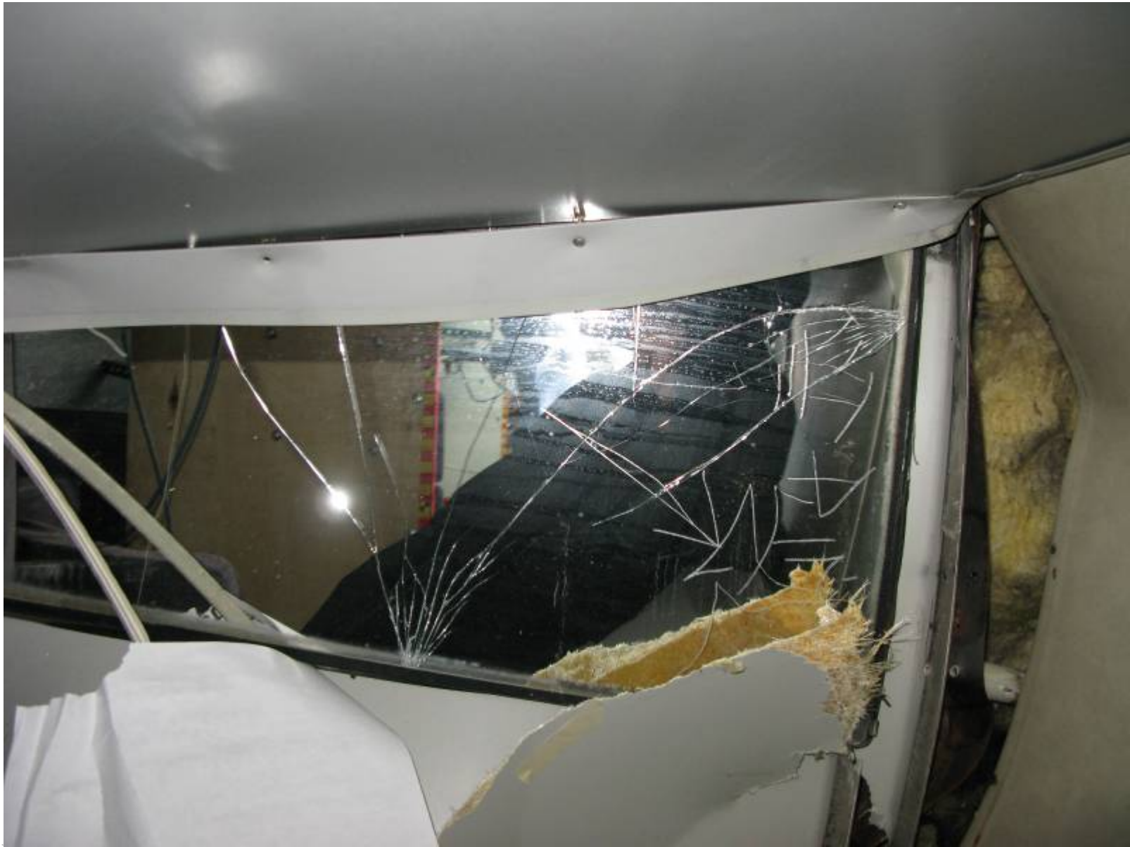
Post-Test Interior Damage View 7
