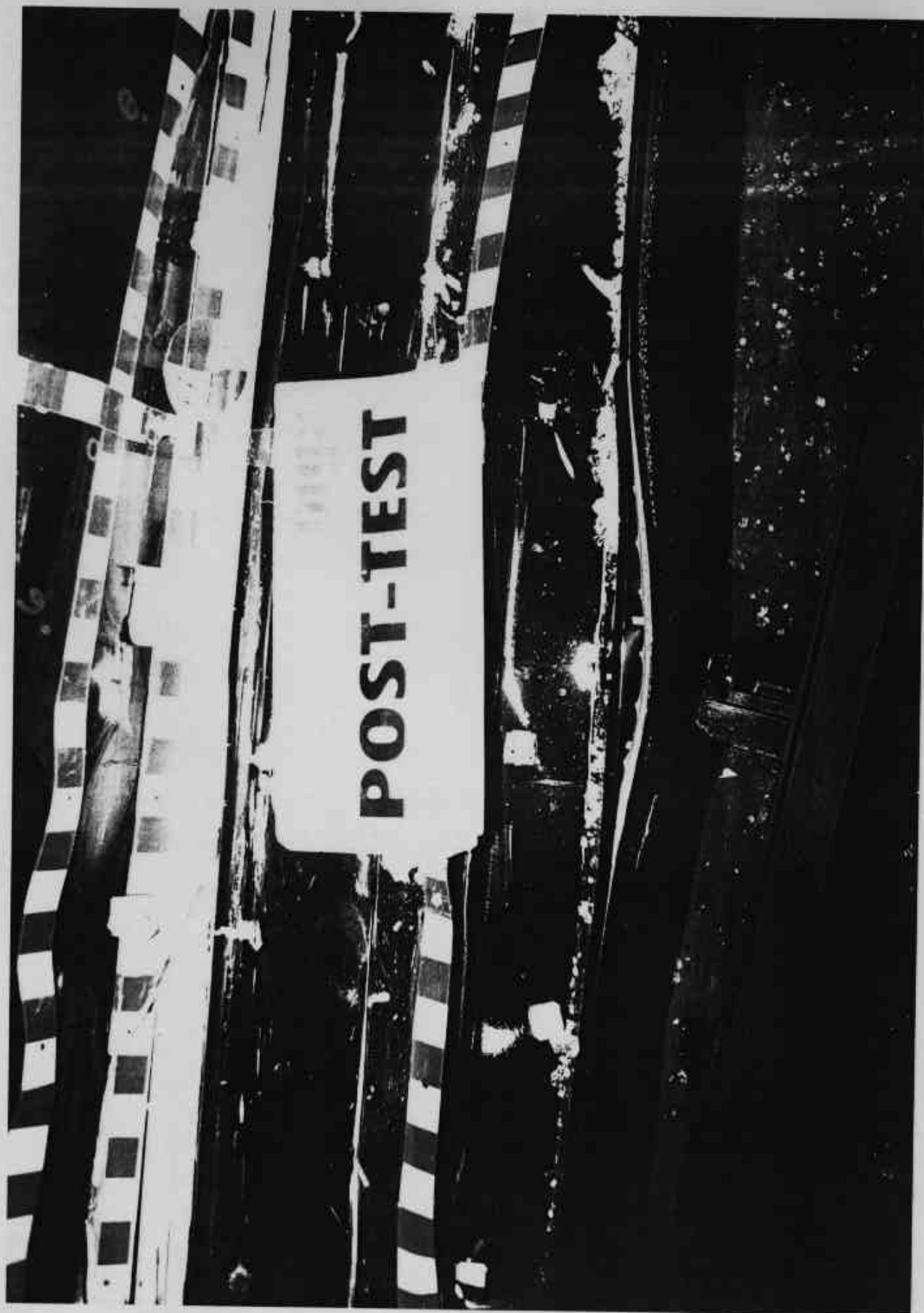
Photo No. A-44 - Sill Separation
