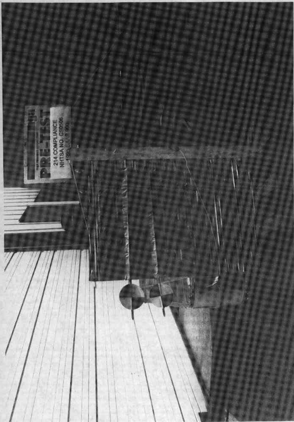
Photo No. A-18 - Pre-Test MDB Left Side View
