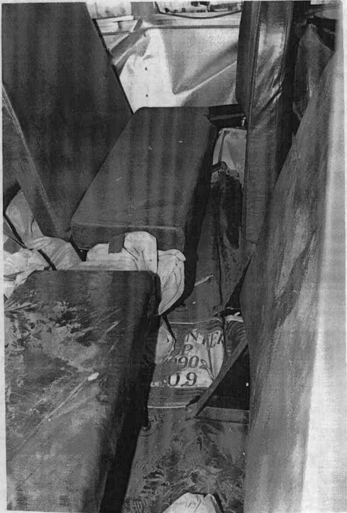
FIGURE 3-8 INTERIOR VIEW OF JOINT SEPARATION - POSTTEST
