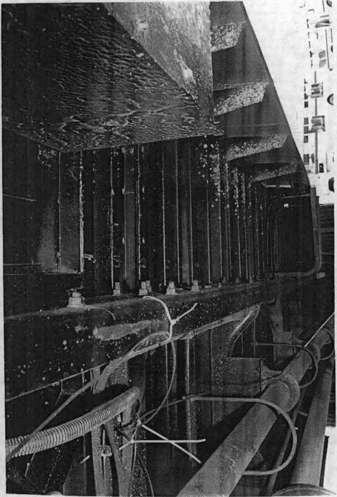
FIGURE 2-6 CLOSEUP UNDERNEATH VIEW OF IMPACT AREA LOOKING FRONT TO REAR - PRETEST
